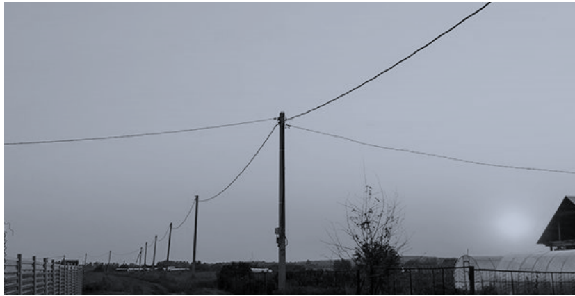
Figure 19 – Catenary Sag of Power Lines
