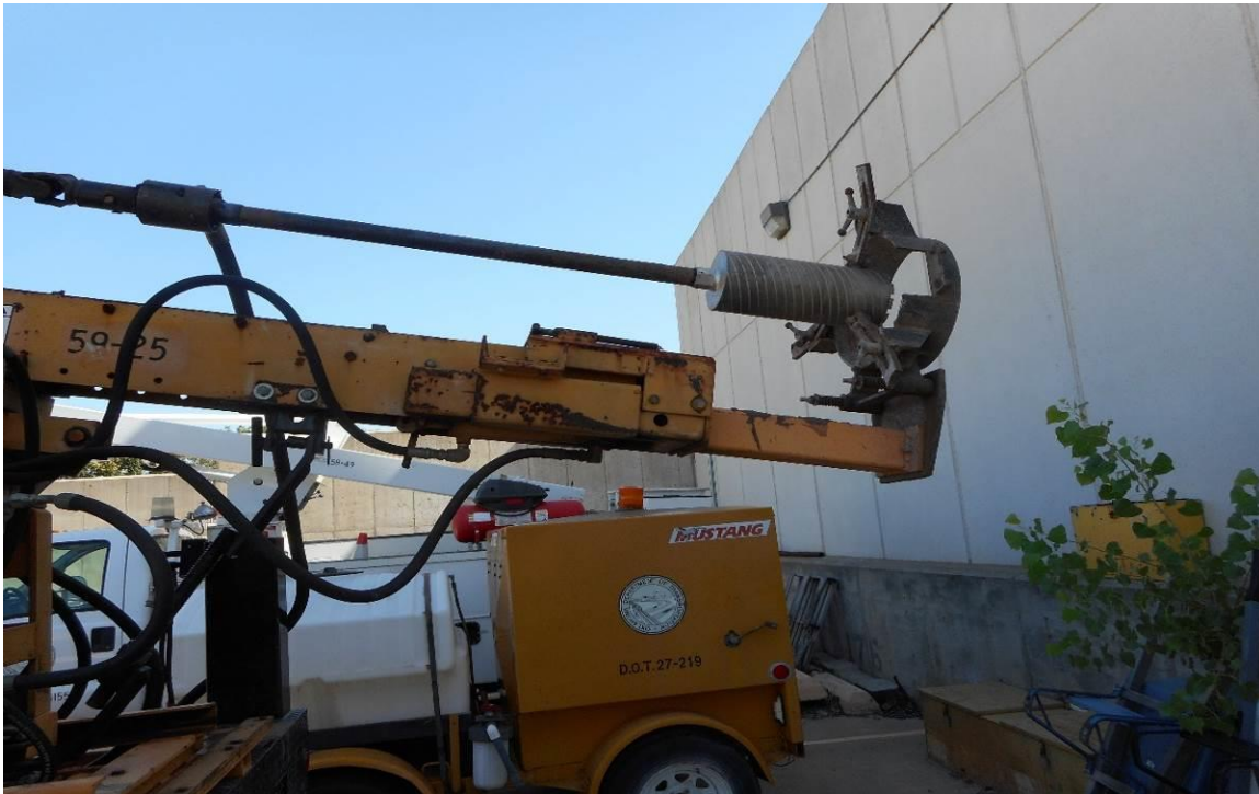
Figure 3.5 Core Bit and Drill Used by ODOT for Extracting the Field Cores
