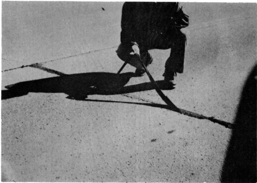
Figure 27. Rubber-Band Type Failure of Synthetic Rubber (Soft) Sealant.
