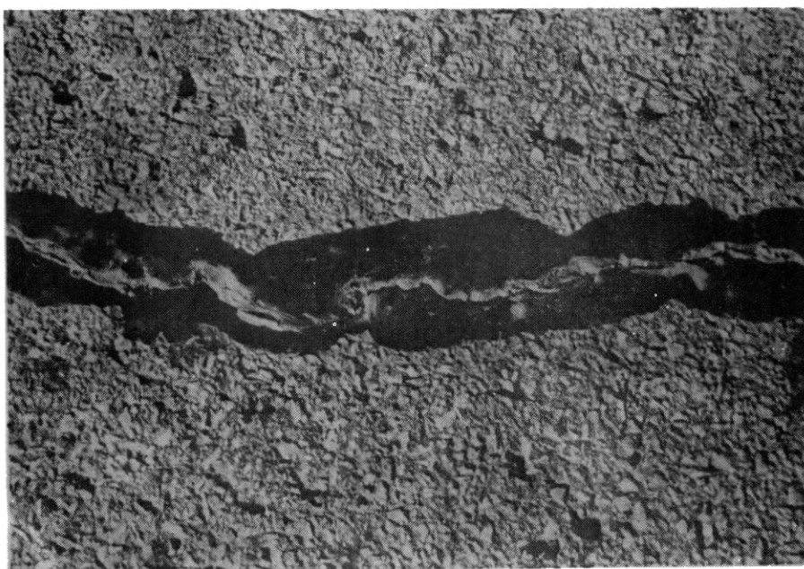
Figure 17. Cohesive Failure of CRS-2 Emulsion.
