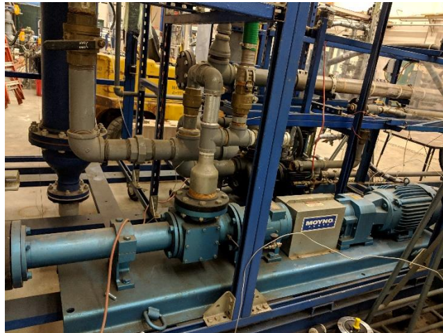
Figure 5. 4: Progressive cavity Moyno pump used to circulate fluids
