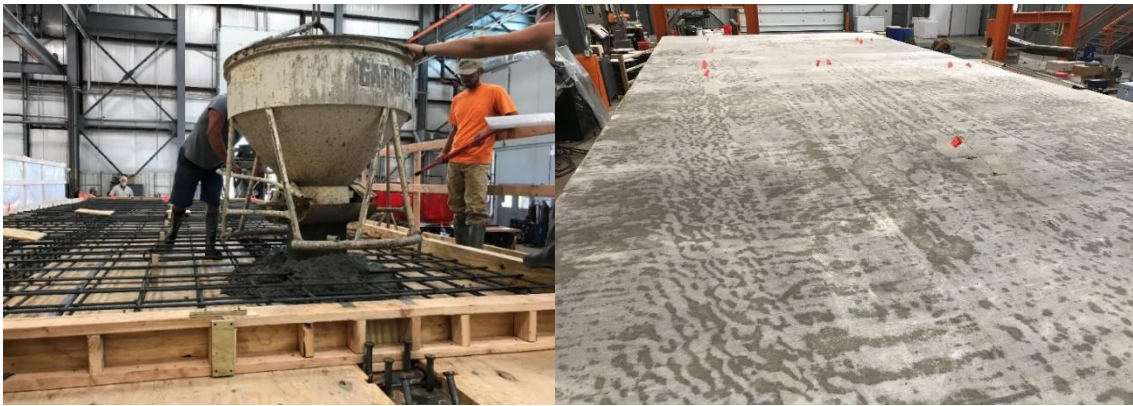
Figure 4.3: Photograph of bridge slab (a) during cast (b) at 14 days after finishing and wet curing with burlap for 14 days
