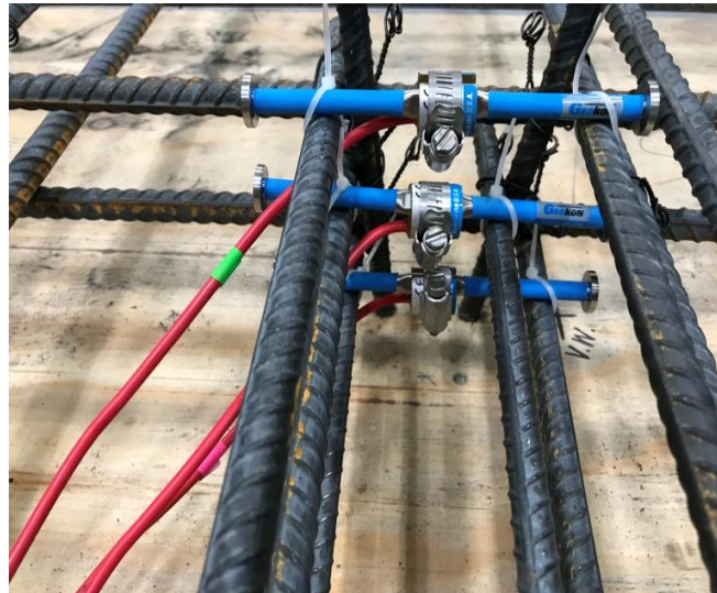
Figure 4.5 - Photographs of VWSG used for data collection: VWSG were placed at depths of 2 in., 4 in. and 6in. prior to slab casting.
