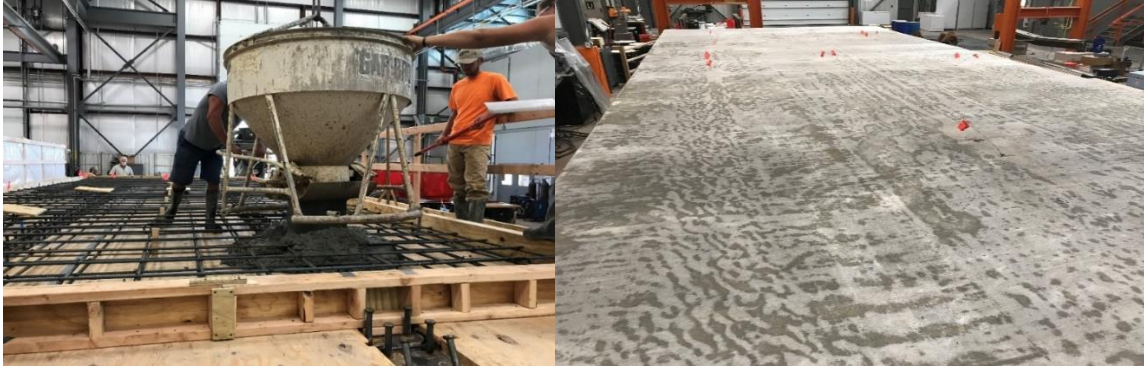
Figure 3.3 - Photograph of bridge slab (a) during cast (b) at 14 days after finishing and wet curing with burlap for 14 days
