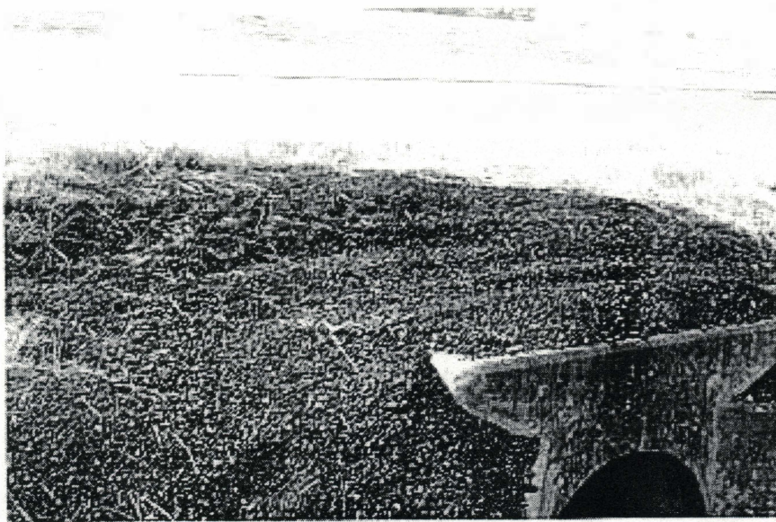
Figure 3.1 Untreated Millings in Erosion Control near I-40 in Sequoyah County
