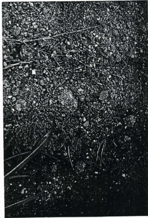
Figure 3.9 Attempted Use of Millings as Ditchliner on SH 18 in Payne County
