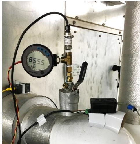
Figure 2.27: Chiller water pressure gauge installation with the Paragon Robotics device to detect the mV output signal from the Omega pressure gauge
