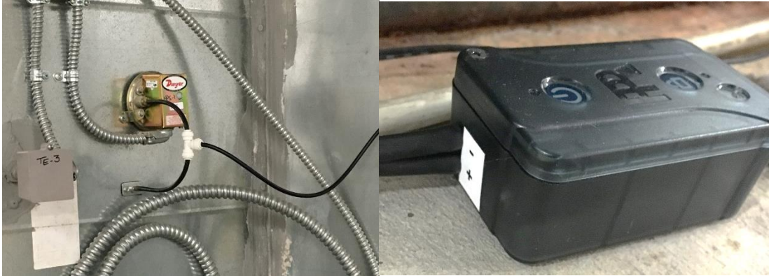
Figure 2.28: SC76 Differential Pressure sensor with two tubes connected. One tube connected to the duct after supply fan into tee tube fitting for negative pressure reading
