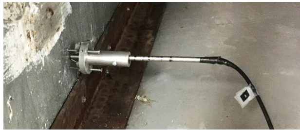
Figure 2.30: TSI air velocity transducer installed in supply ductwork
