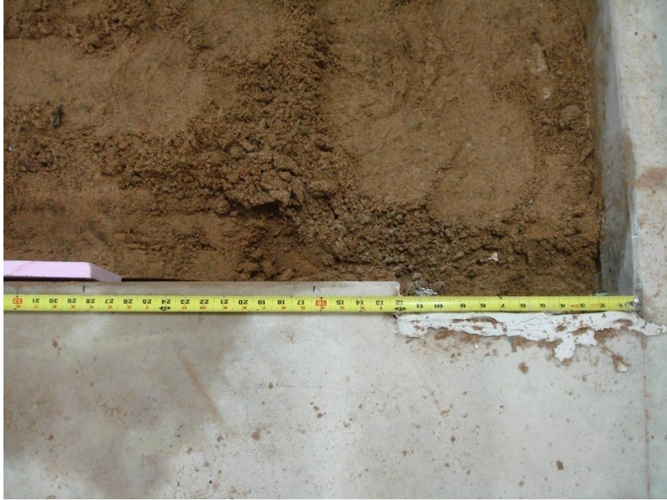
Figure D.3 Making measurement for the end of slab to provide 9 in. depth
