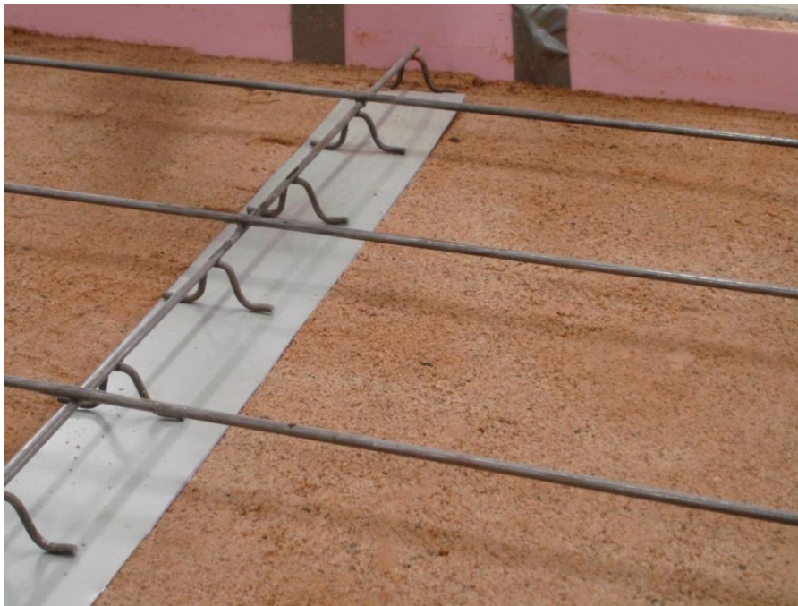
Figure D.8 Chair placed on the Aluminum sheet to prevent depressing chair into the sand
