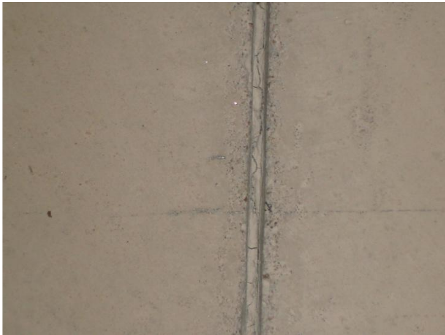
Figure 4.9 Top View of joint opening expansion or crack at large scale slab specimen
