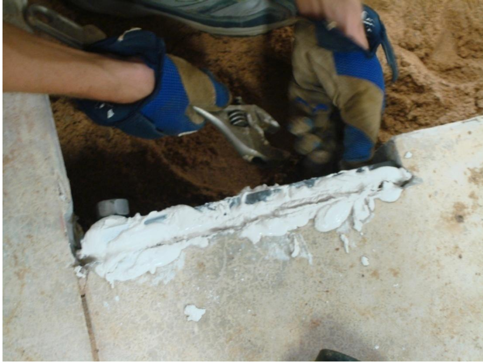
Figure D.7 Fixing location of the plate at the end of the slab specimen
