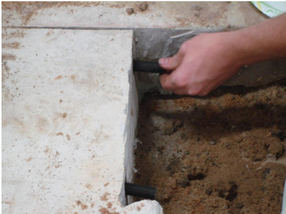
Figure D.4 Placing bolt into the existing slab floor at the end of slab specimens
