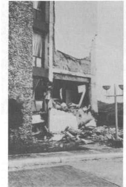
Figure 5.3. Failure of lower level of masonry-infilled reinforced concrete frame (Paulay 1992)
