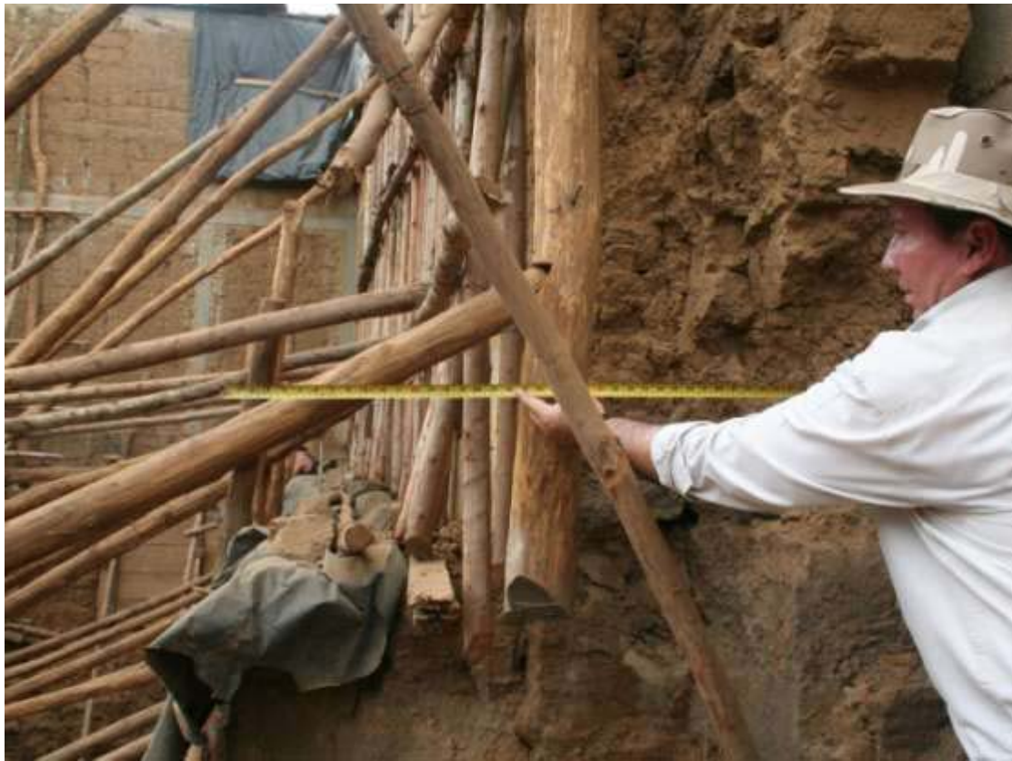
Figure 7.3. Construction manager in front of the collapsed adobe wall
