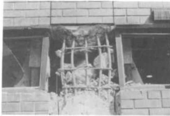
Figure 5.5. Short column failure (Paulay 1992)
