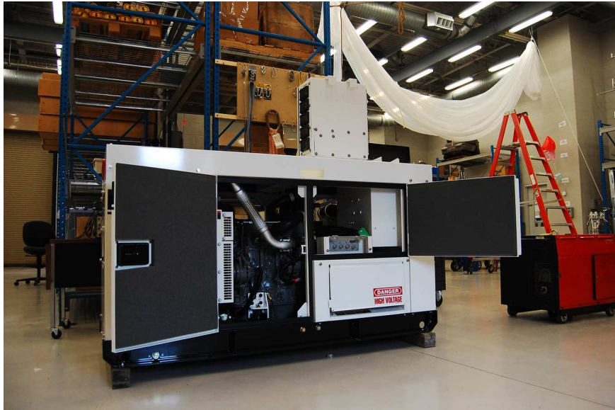
Figure 4.16: An image of the 20-kW diesel generator that provides electrical power to the AIR. Power output is 240 VAC single phase and passes through a transfer switch prior to entering the main breaker box, which distributes power to the subsystems.
