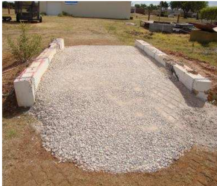
Figure 7.30. The top (second) layer of aggregate in the test bed after compaction
