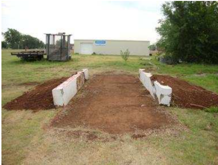
Figure 7.20. Concrete beams placed on both sides of the test section with soil support on the outside
