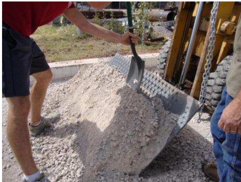
Figure 7.33. Tilting of steel plates and removing of aggregates to facilitate exhumation process
