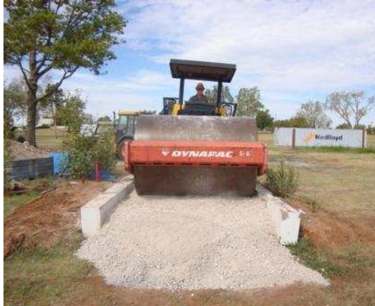
Figure 7.29. Compaction of the second layer of aggregate with the vibratory roller compactor
