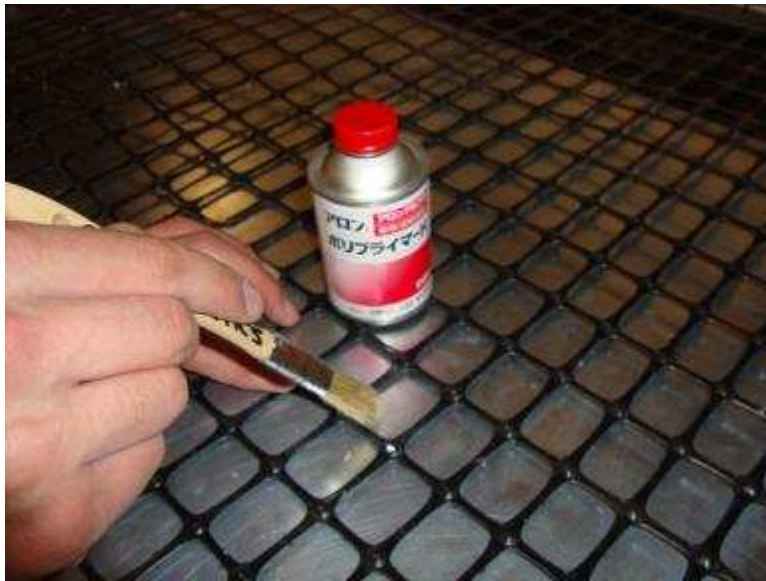
Figure 9.11. A brush was used to remove dust due to abrasion
