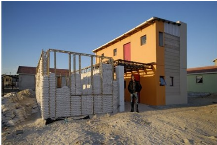
Figure 8. MMA's Indaba House features a two-story timber frame with sandbag infill in Cape Town, South Africa
