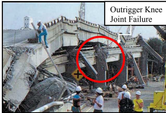
Figure 1.2: Collapse due to outrigger knee joint failure during 1989 Loma Prieta Earthquake (Wikipedia, fn. USGS)
