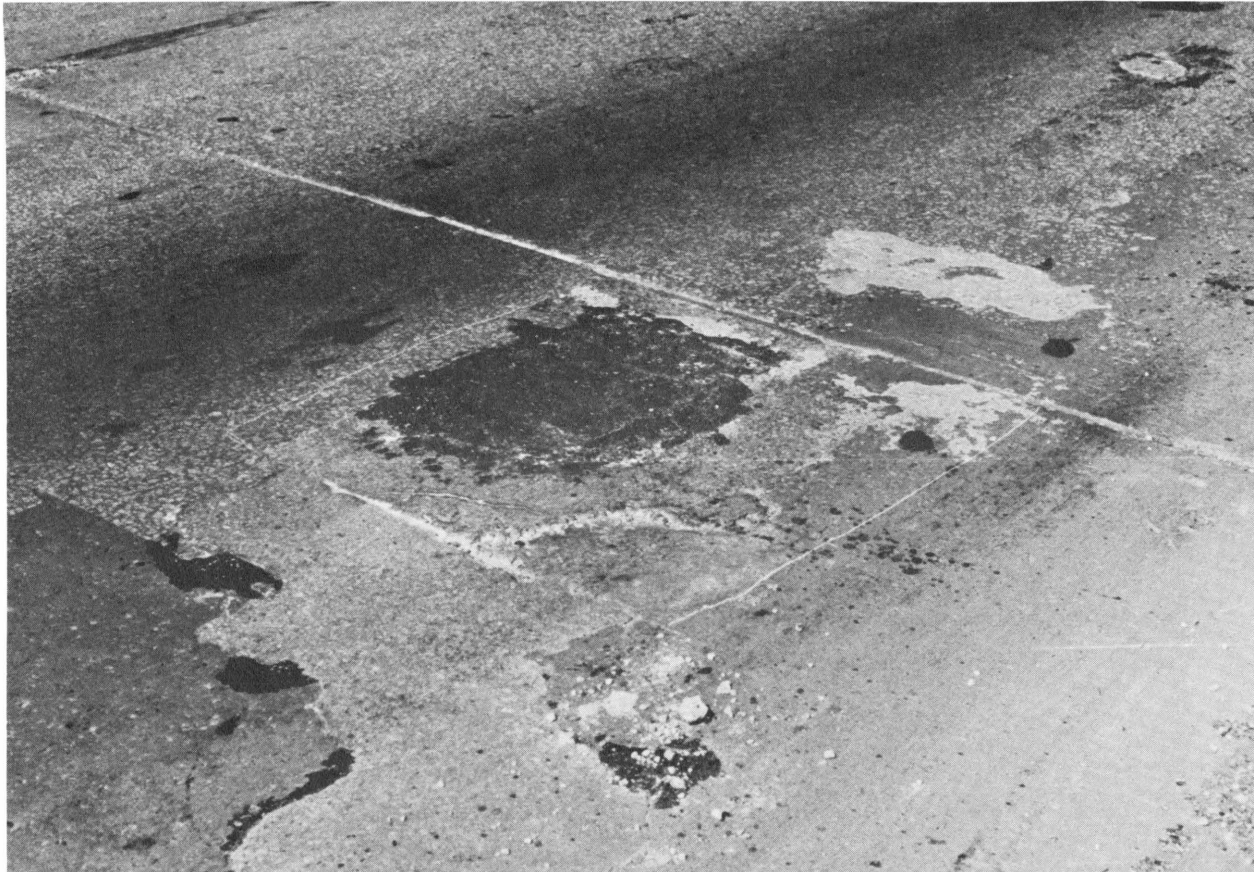
Figure 1.1 A Damaged Bridge Deck with Potholes
