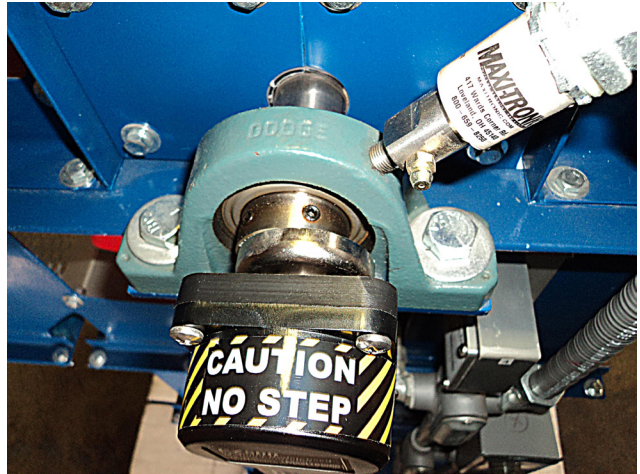
Figure 9. Bearing temperature sensor and shaft motion sensor.
