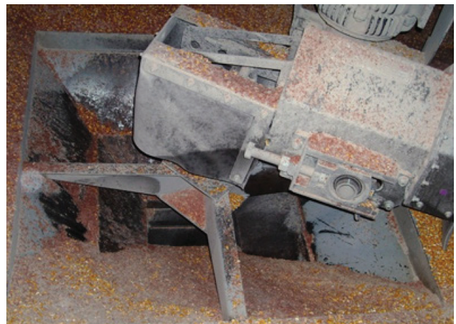
Figure 2. Unguarded bin sump.
