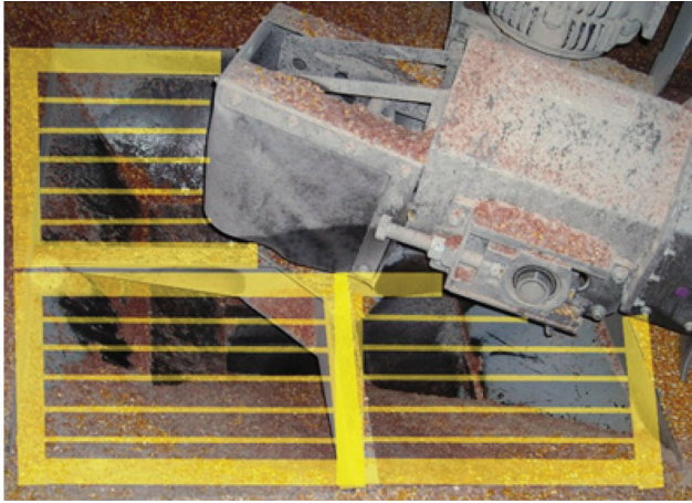
Figure 3. Guarded bin sump.
