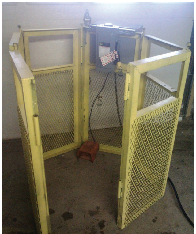
Figure 12. Worker protection caging and sweep auger controls.
