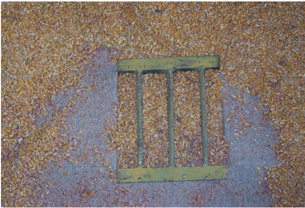
Figure 4. Improperly secured grate.
