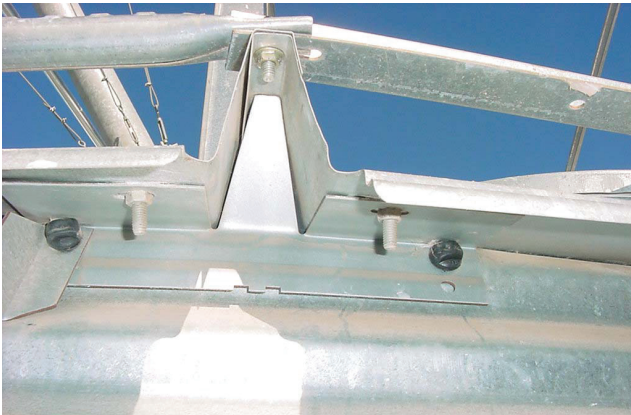
Figure 10. Roof panel stiffening rib fitted with a metal plate. Caulk cracks around the edges of the plate from inside or outside the bin.
