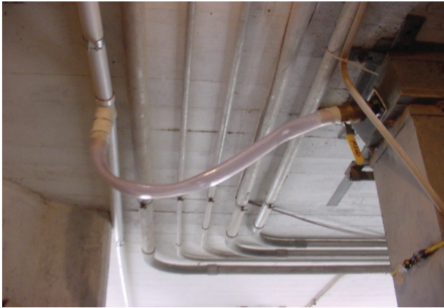
Figure 4. CLF injection point with ball valve into discharge spout of concrete elevator bin.
