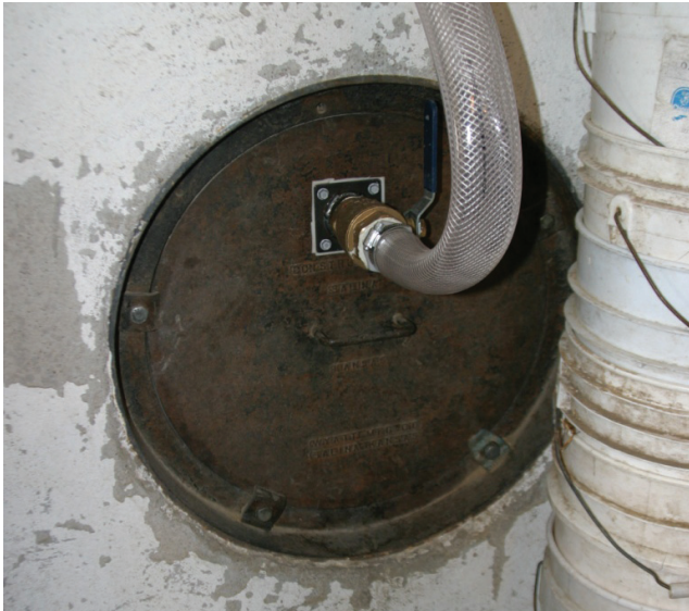
Figure 3. Manhole cover in concrete silo with CLF injection point and ball valve to isolate bin.
