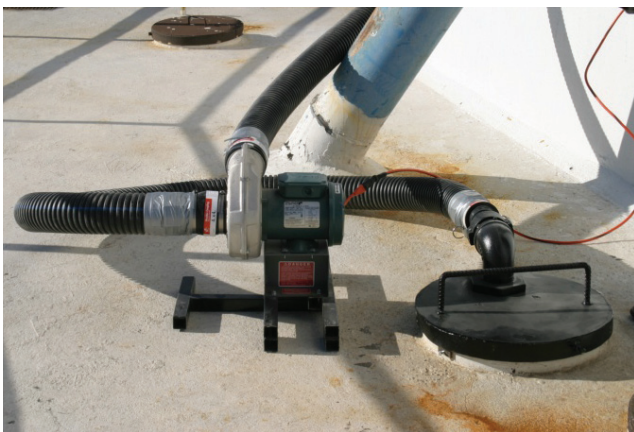
Figure 5. CLF fan pulling gas through manhole cover on top of concrete silo. Flexible corrugated drain hose is used for temporary connections.
