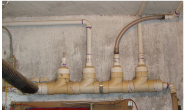
Figure 7. PVC distribution manifold for CLF system.
