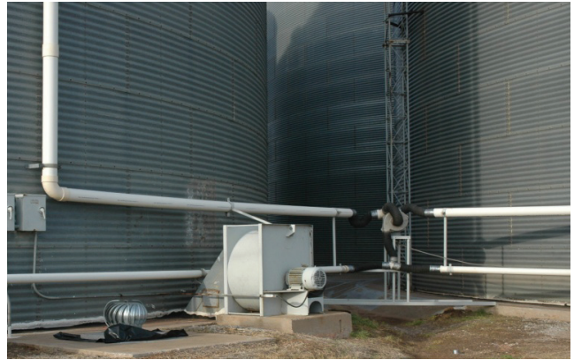
Figure 6. CLF system on steel bins.
