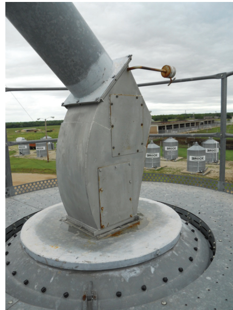
Figure 13. Fill spout equipped with a self-closing door to reduce leakage up the leg. Seam where fill spout attaches to top of the bin needs to be caulked also.
