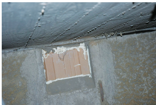
Figure 8. Sealing concrete silo top vents with closed cell expandable foam. Interior cardboard support is temporarily held in place with wire while foam is applied from outside.
