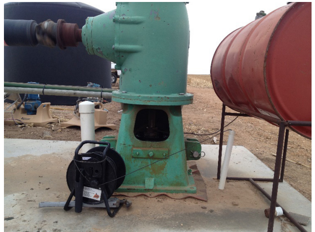
Figure 3. Cable going into well access tube.
