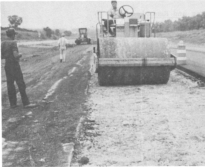
Figure 6. The cracked pavement was rolled with a steel wheeled roller to ensure seating.
