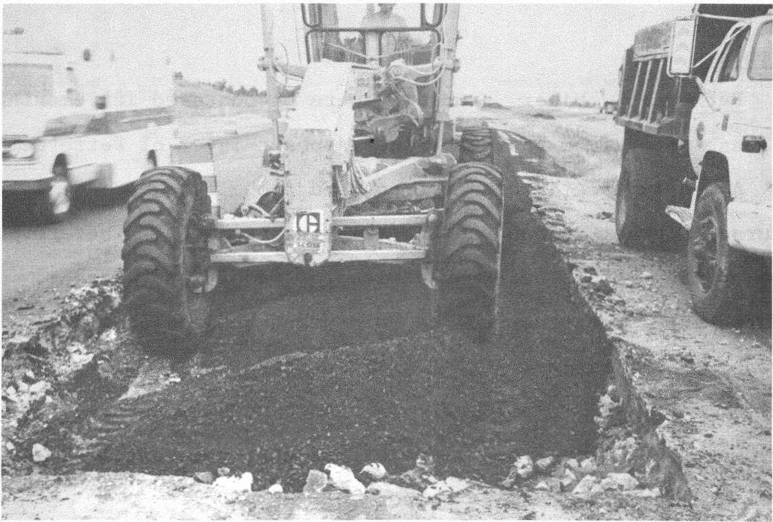
Figure 8. A PCC pavement section. It was removed and patched with full depth Type A AC mix.
