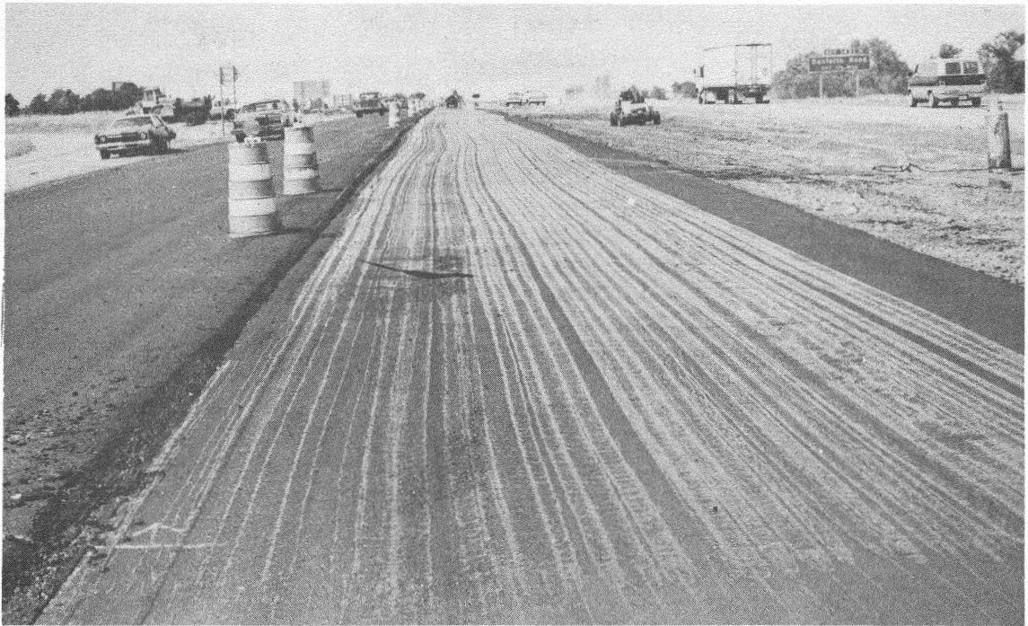
Figure 10. The tack coat was not spread uniformly due to a faulty asphalt distributor.
