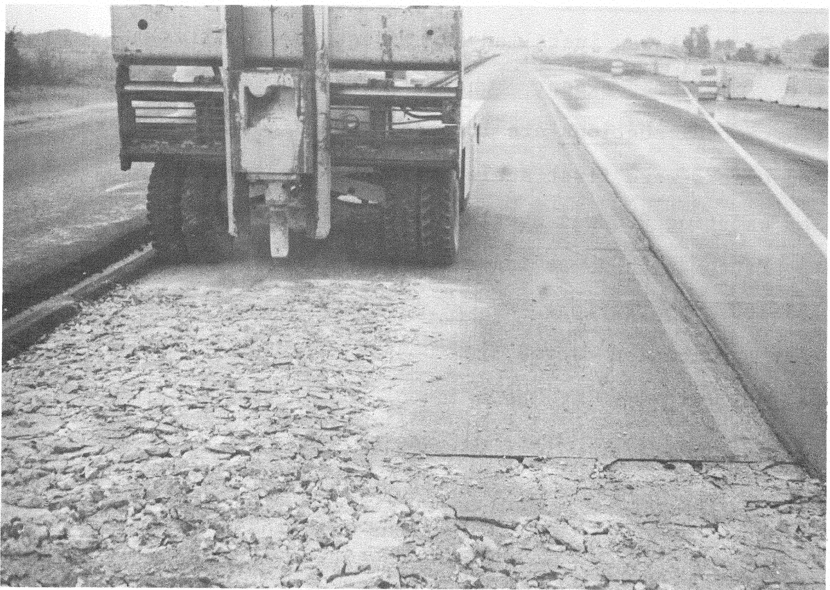
Figure 5. The existing slabs were cracked with a pile driver type pavement breaker where removal or seating was desired.
