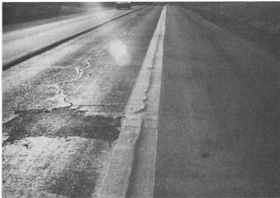
Figure 3. Polyguard strip membrane installed over the longitudinal edge joint between the PCC slab and AC widening section.
