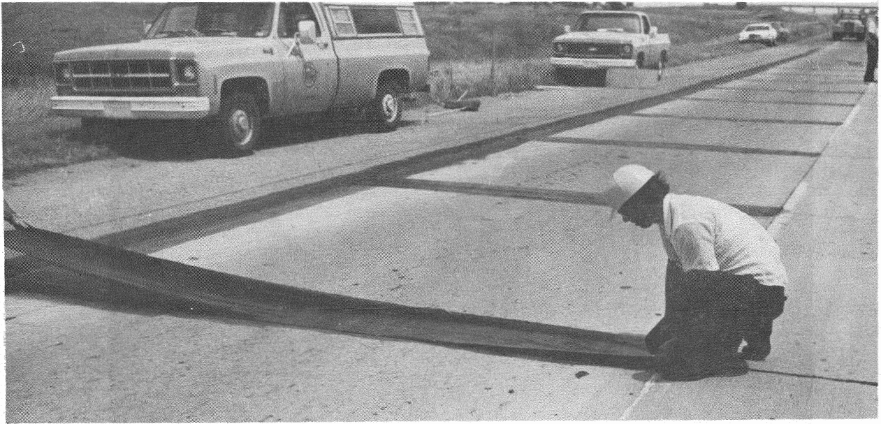
Figure 6. All the transverse, centerline and outside longitudinal joints were covered with 1.5 ft wide Bituthene on the northbound lanes.
