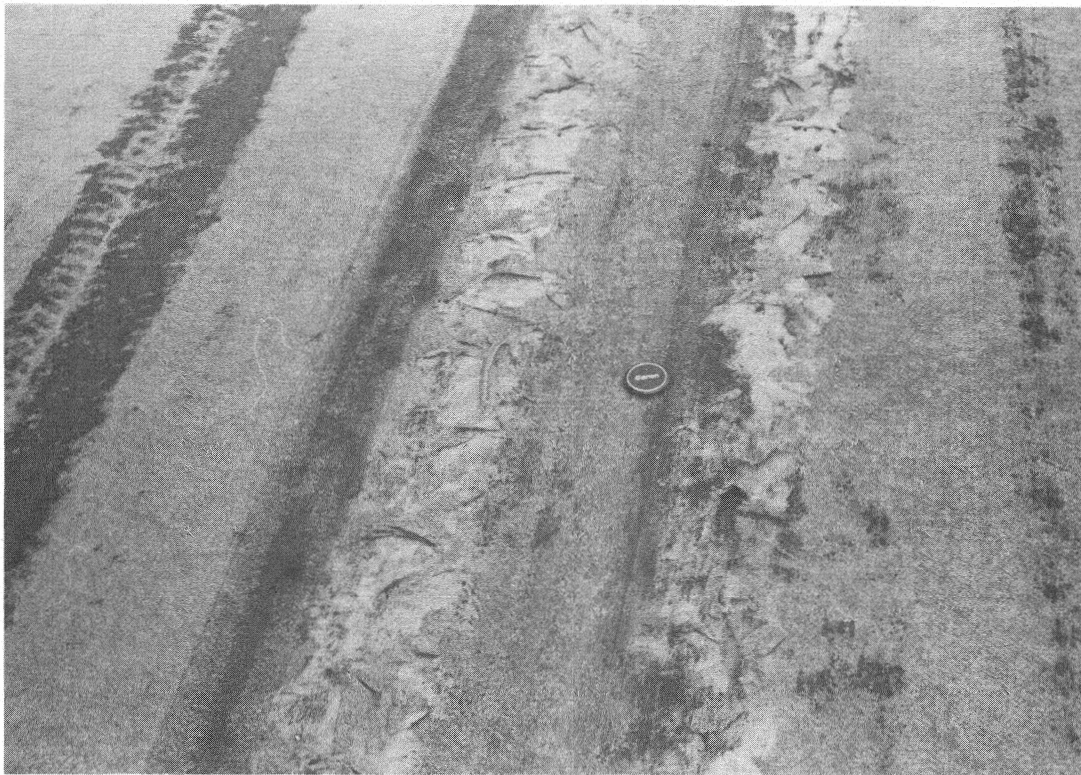
Figure 13. View of disturbed Petromat.
