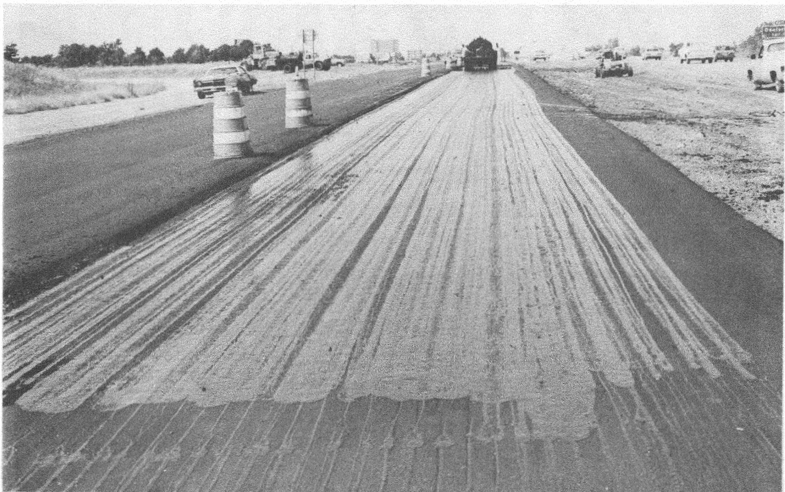
Figure 11. The tack coat for the Petromat was applied twice in order to get even coverage.
