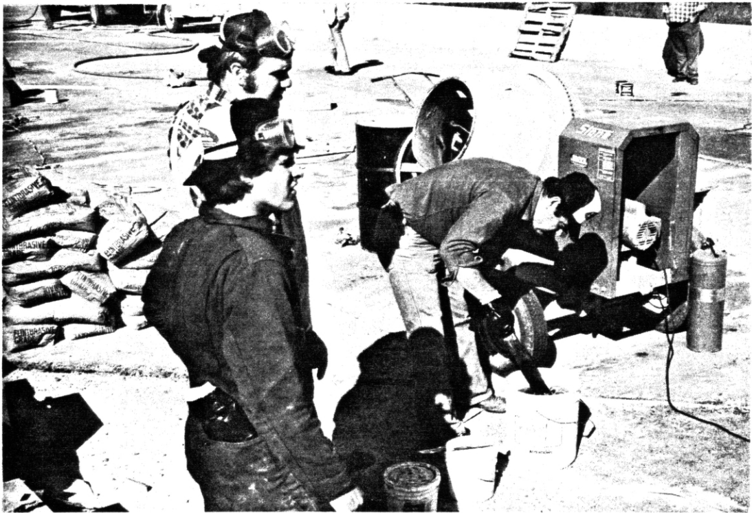
Figure 22. For patching, polymer concrete was mixed with a portable mixer and placed by hand.
