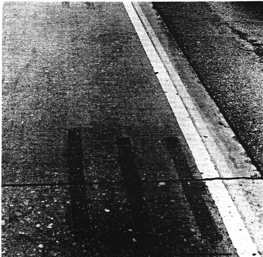
Figure 8. Distressed Dowel Bar
