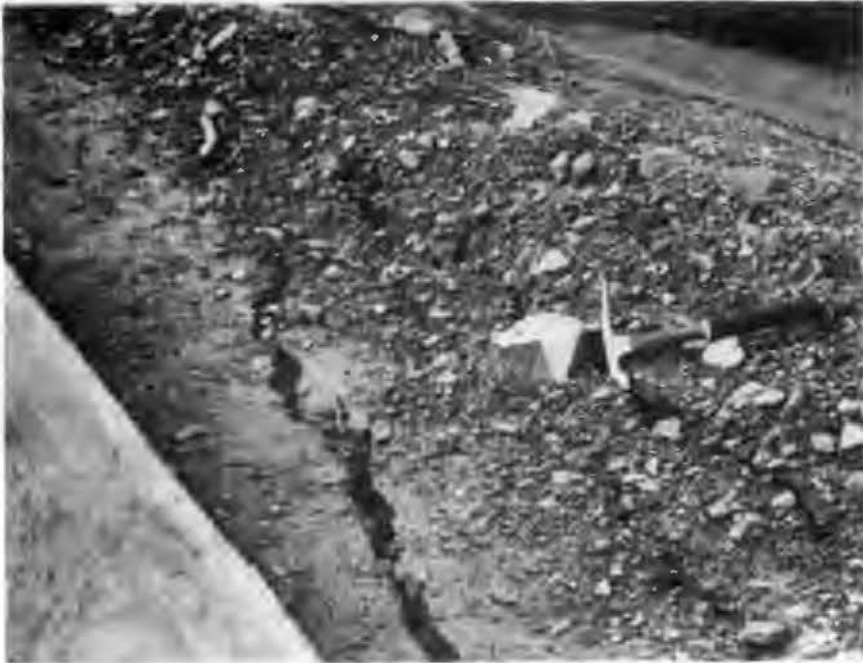
Figure 15. Tension cracks along the front edge of the upper embankment of the road built on the escarpment of Norristown Mountain (NE \frac{1}{4} sec. 17, T7N, R20W).
