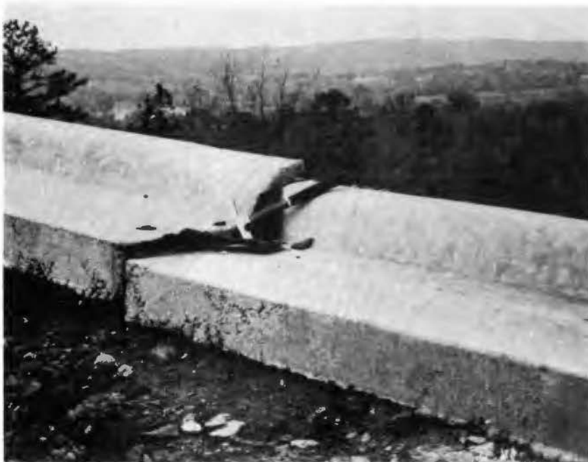
Figure 14.- Vertical misalignment of curbs due to slope instability on the escarpment of Norristown Mountain (NE \frac{1}{4} sec. 17, T7N, R20W).
