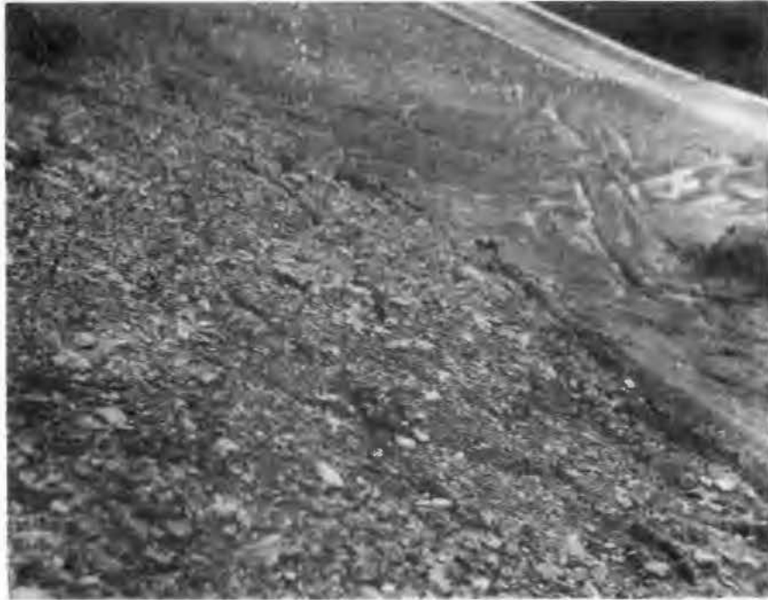
Figure 16. - Tension cracks in the Atoka Formation shale exposed in the backslope of the roadcut across the Norristown Mountain escarpment (NE \frac{1}{4} sec. 17, T7N, R20W).
