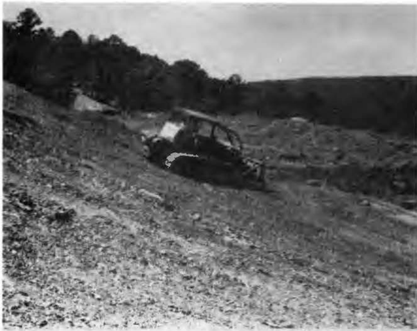
Figure 13. - Construction of the roadway on the Norristown Mountain escarpment (NE \frac{1}{4} sec. 17, T7N, R20W).
