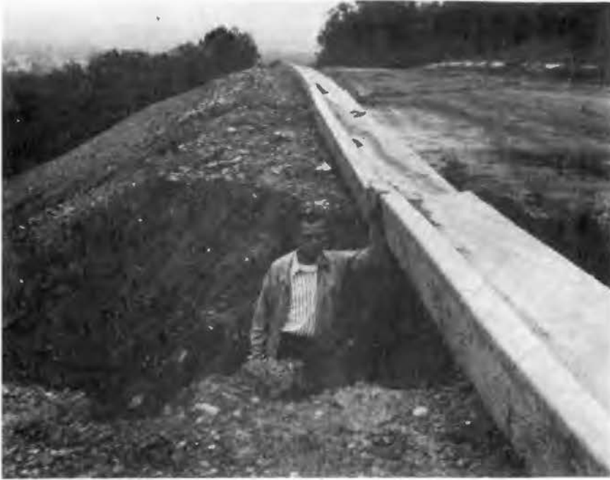
Figure 17. - Erosion caused by inadequate storm drains in the roadway built on the escarpment of Norristown Mountain (NE \frac{1}{4} sec. 17, T7N, R20W).
