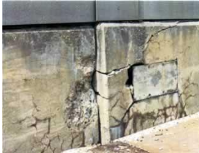
Figure 1: Concrete damage caused by alkali-silica reaction. 7
