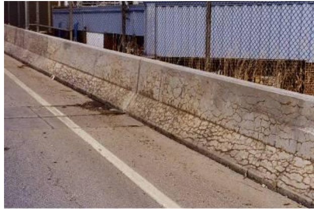
Figure 1: ASR cracking on a bridge parapet in Illinois. 3
