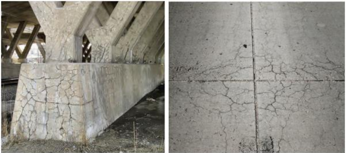
Figure 2: Extensive ASR cracking found in bridge columns (left). ASR damage in pavement slabs (right). 4
