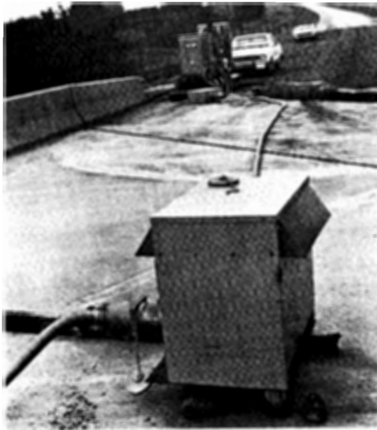
Photograph 13: Transformer with the fuse box and generator in the background.
