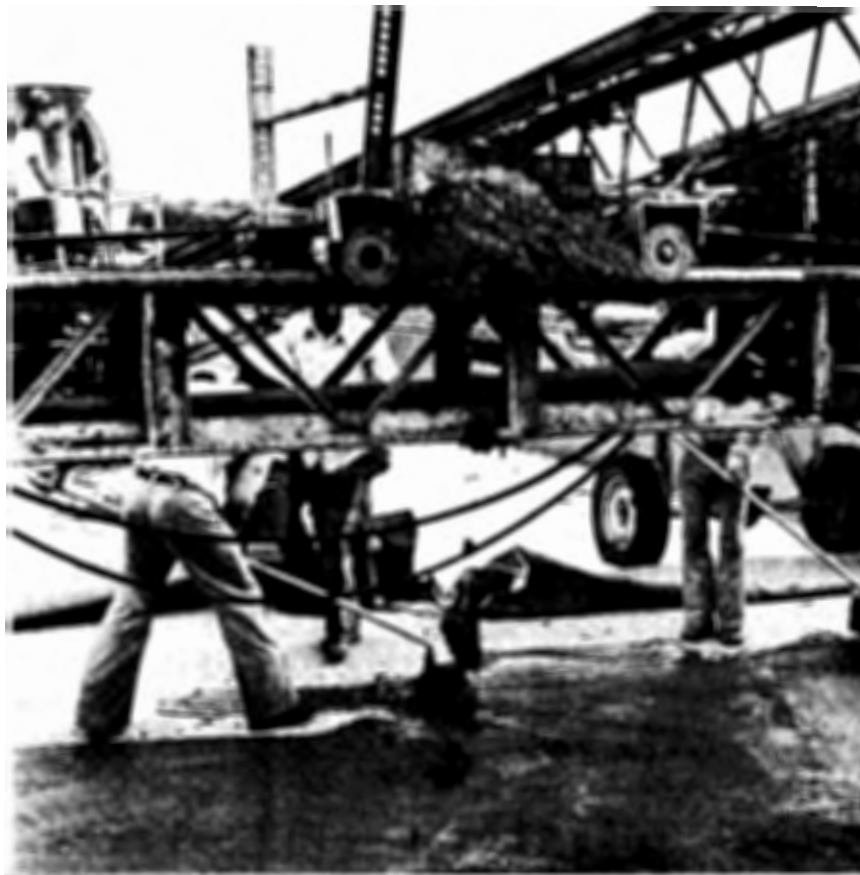
Photograph 8: A sand-cement grout was broomed on the bottom course immediately before the wax bead overlay was placed.
