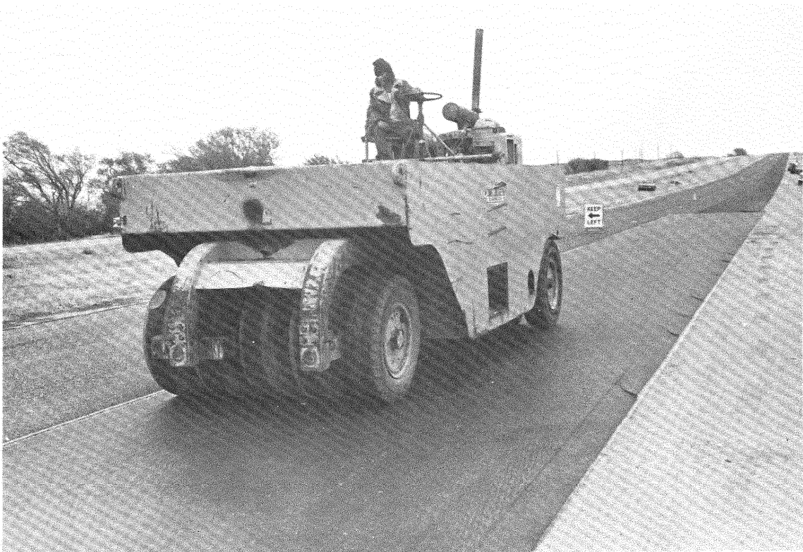
Figure 7 and 8. The recycled overlay was placed in a conventional manner. No special equipment was required.
