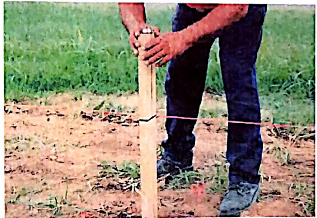
Fig. 4d: Using bubble level and string line to set post position and alignment.
