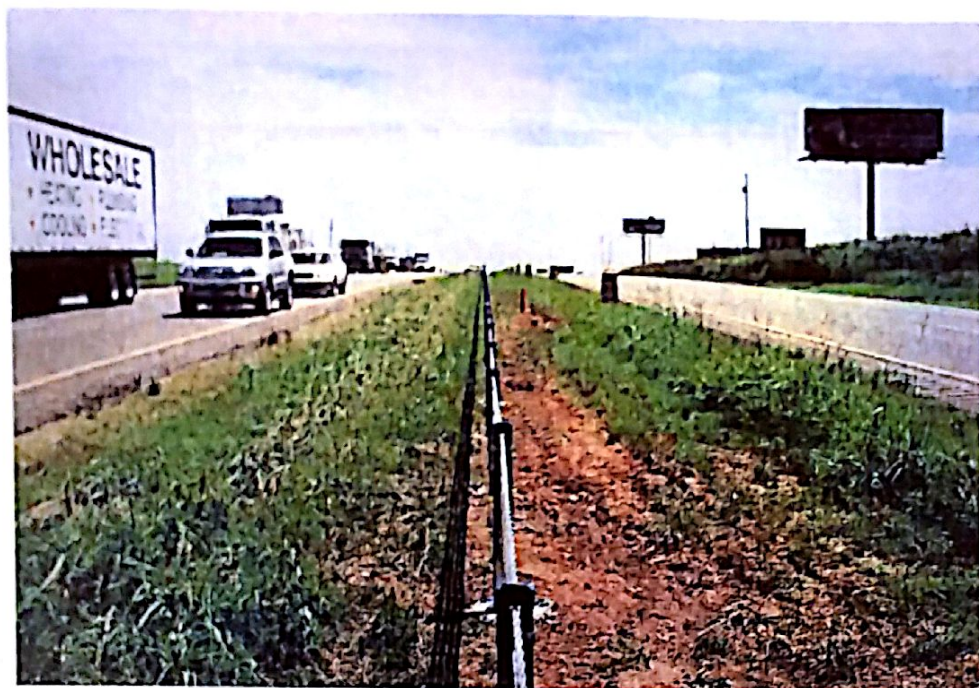
Fig. 5m: Fully assembled and tensioned Safence Cable Barrier System in place on I-35 in Mc Clain County.
