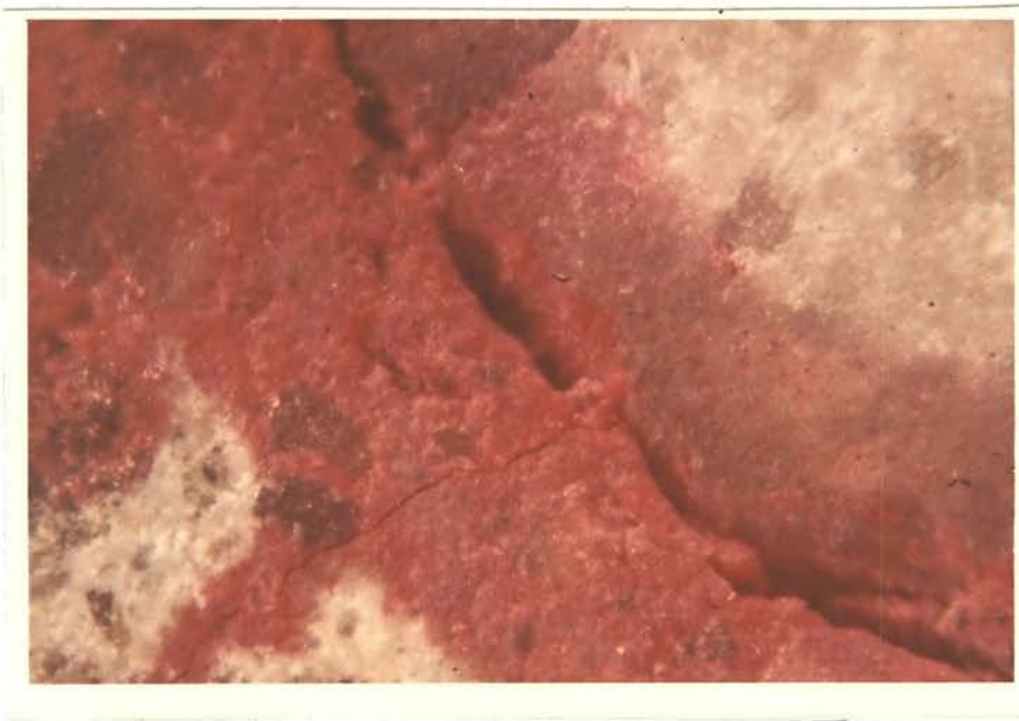
Figure 13. Aggregate Bond Crack and Matrix Crack on Core Sample Similar to A1, A2, A3. Damage was Done Eight Years Prior to Photograph. Magnification is 51x
