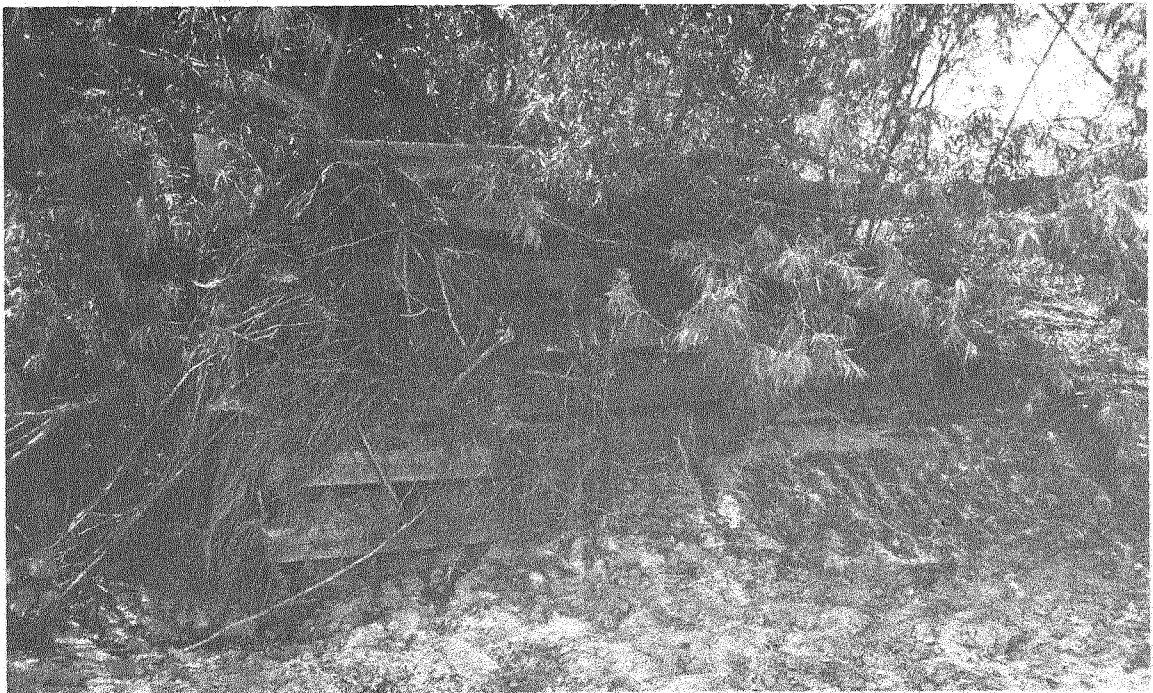
Second Pile Diversion in a Deteriorated Condition
