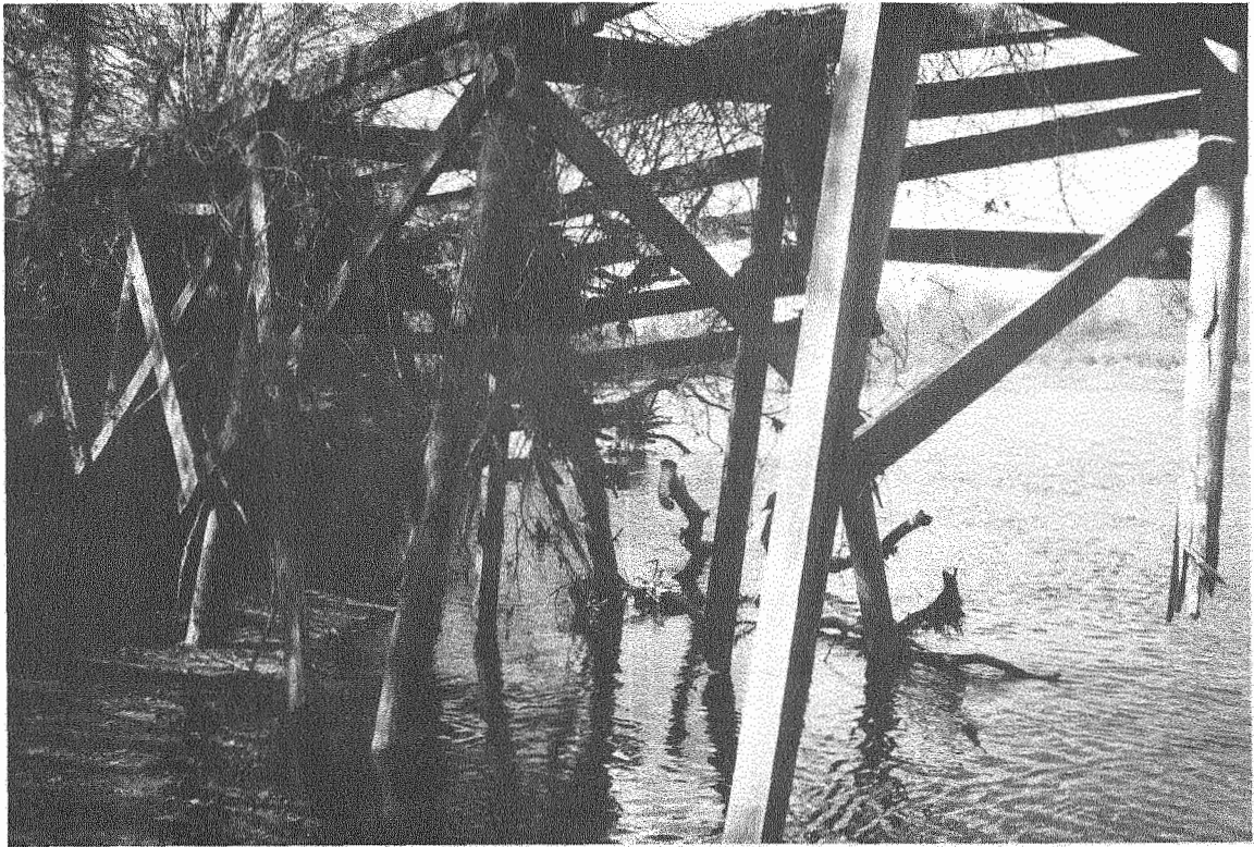
View of Damaged Pile Diversion
