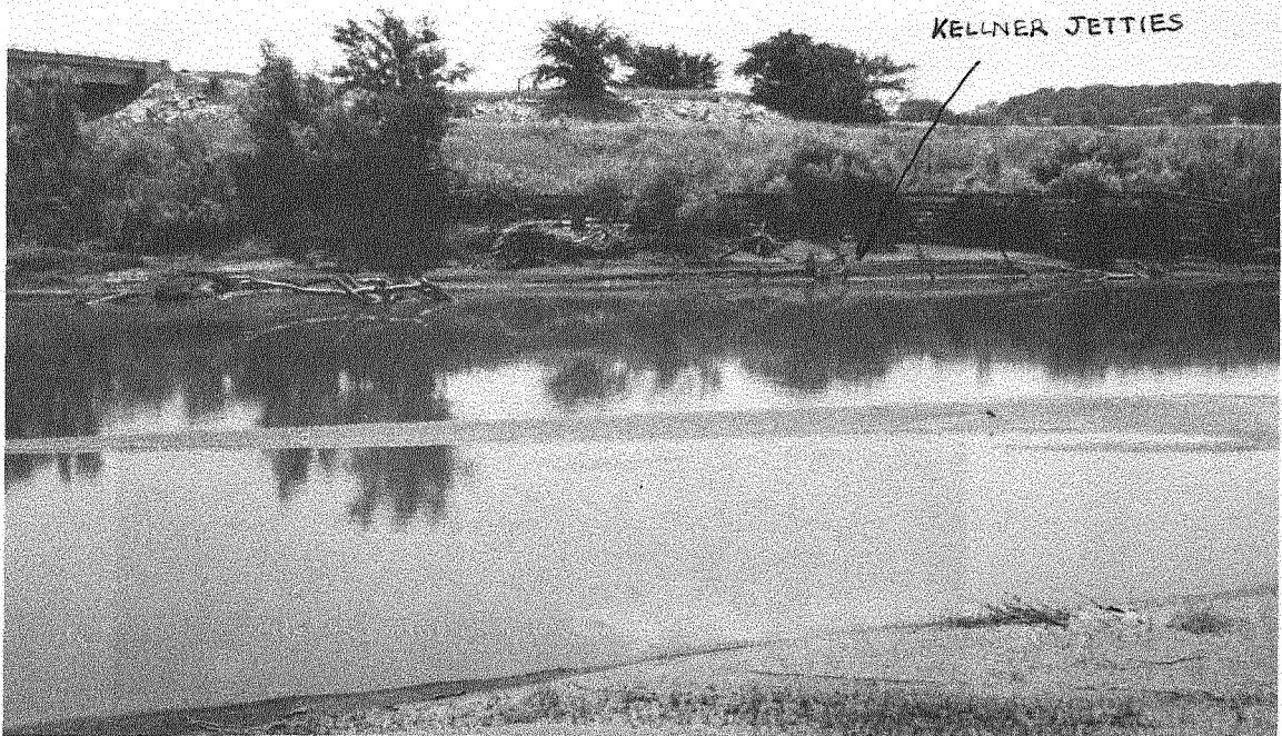
Damaged Pile Diversion
