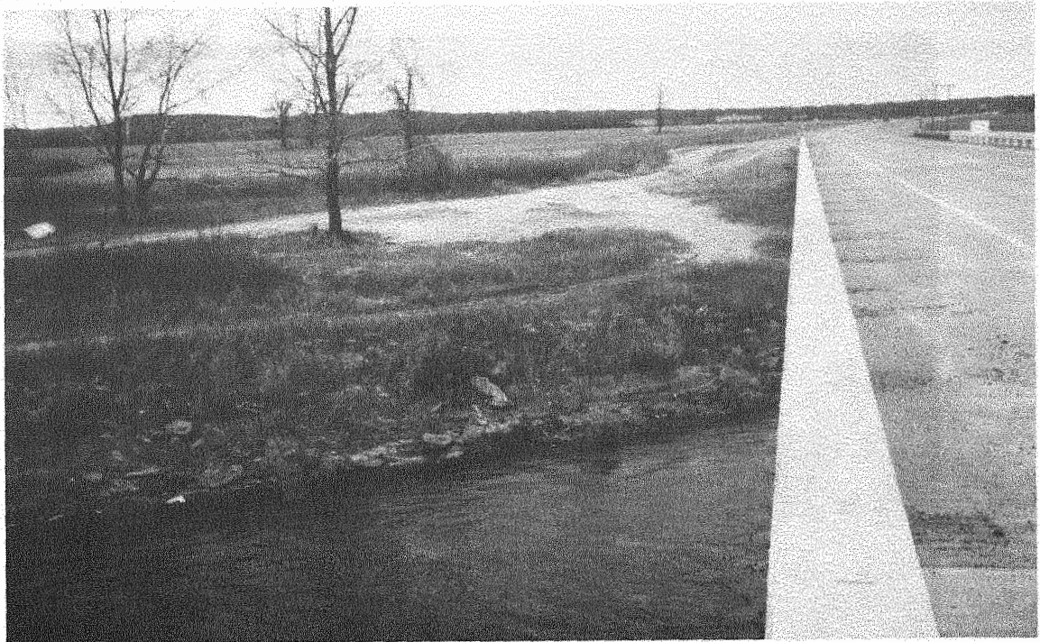
Damaged Riprap at Bridge Abutment
