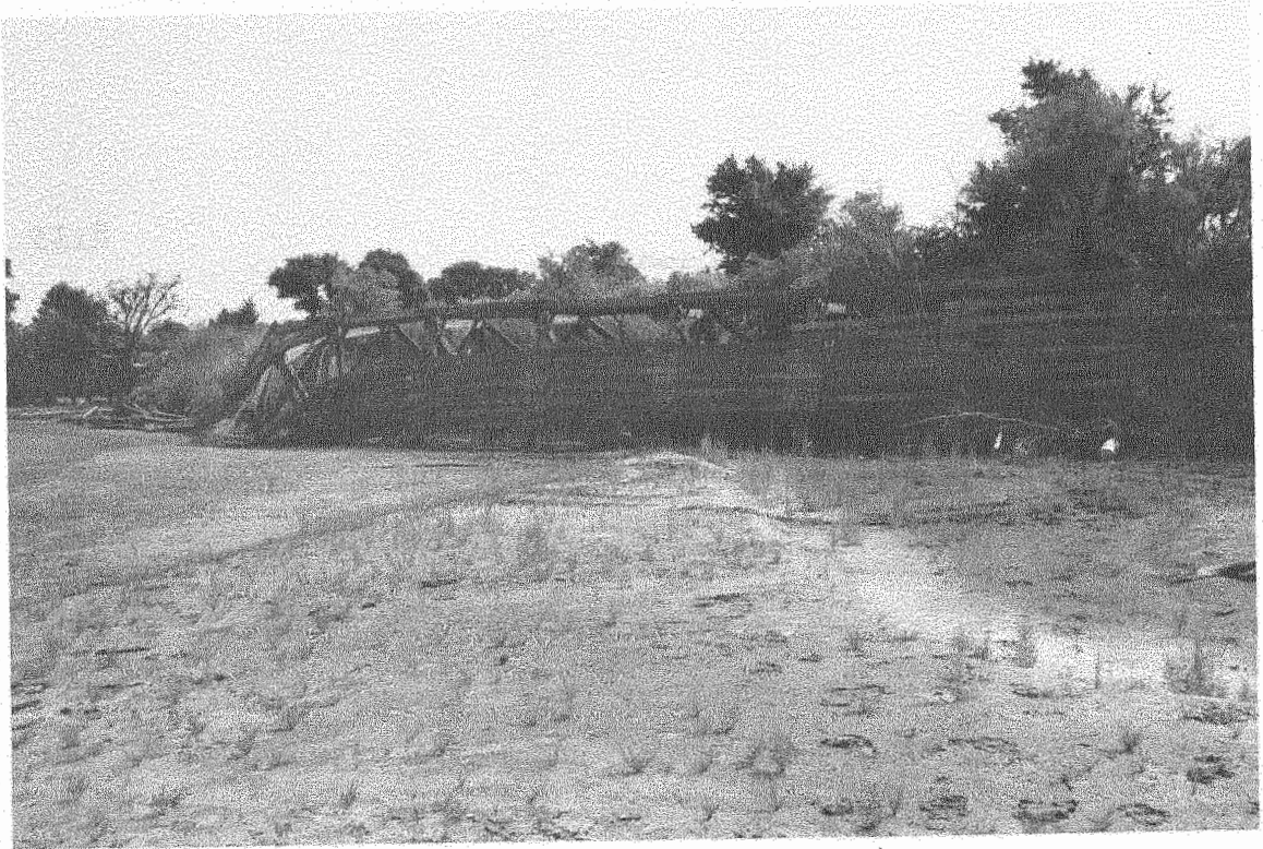
Pile Diversion with Missing Face Planks
