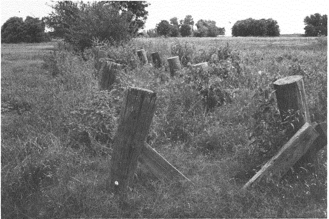
VIEW OF DAMAGED PILE DIVERSION FIGURE 31c
