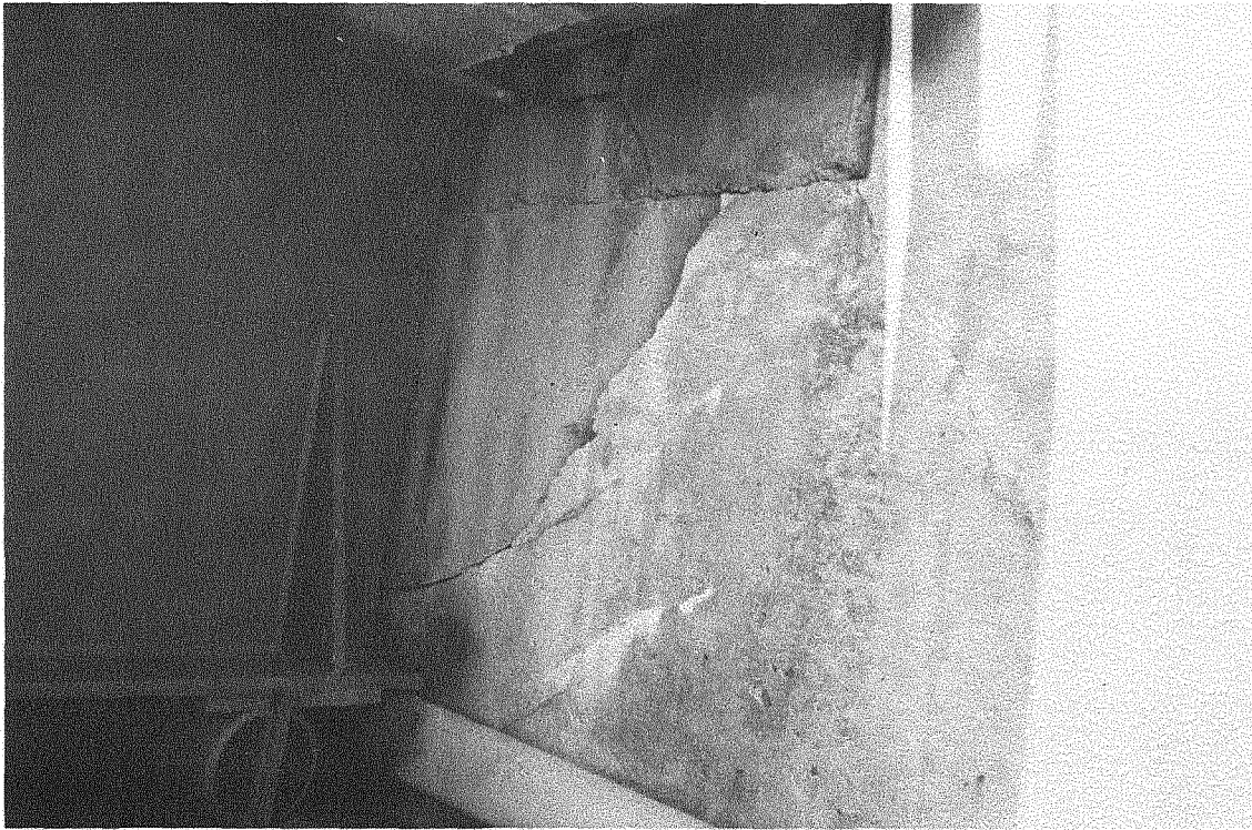
Fig. 2-17. An abutment headwall showing moderate cracking
