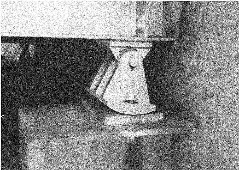
Fig. 2-20. Expansion device showing moderate tilting
