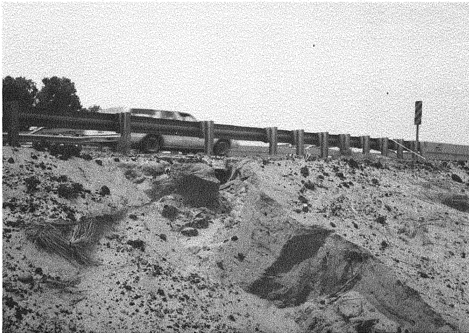
Fig. 2-11. An approach embankment showing erosion
