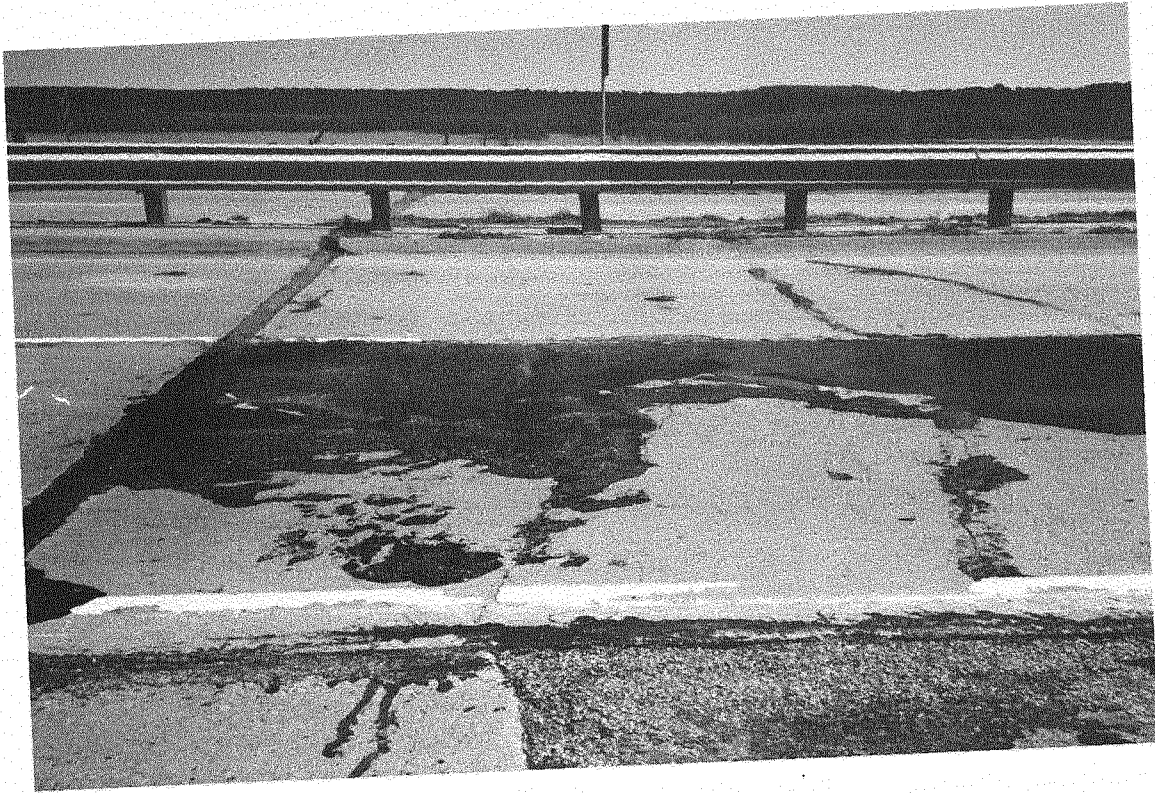
Fig. 2-8. A rough bridge approach
