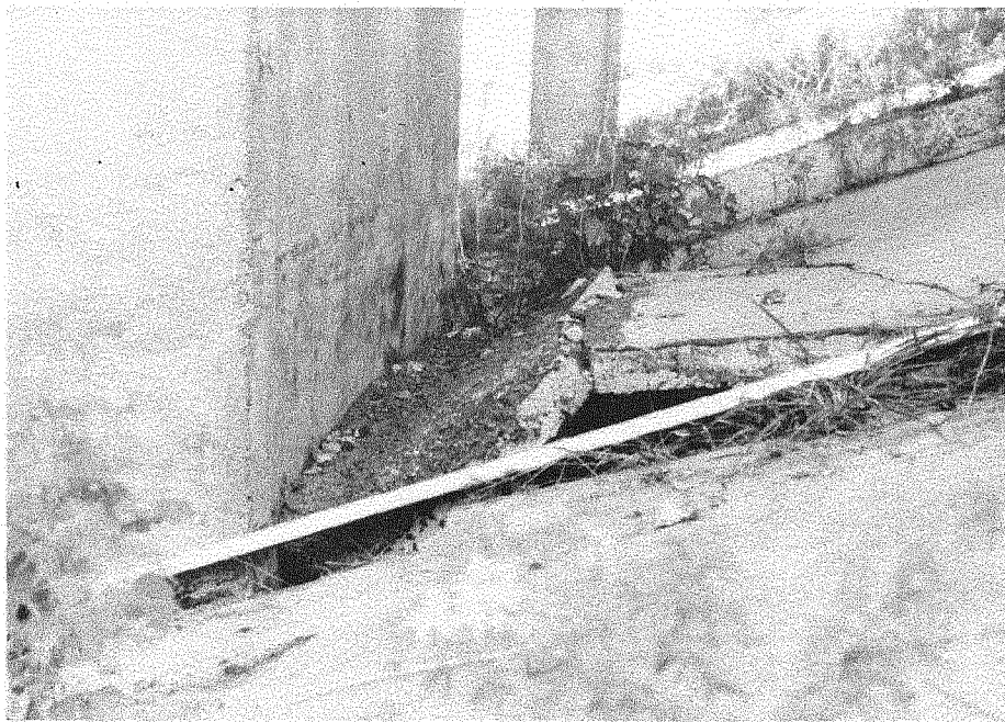
Fig. 2-10b. A slope protection structure showing extensive cracking and settlement
