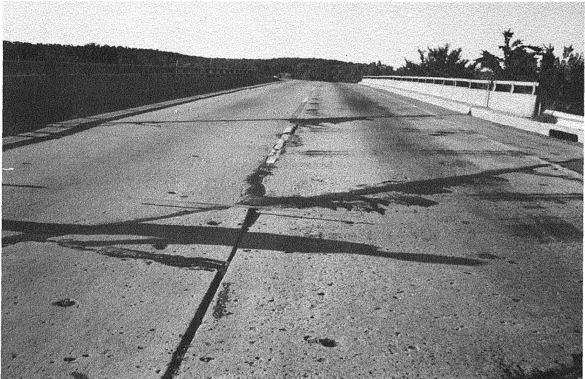
Fig. 2-22. Differential settlement between truck lane and nontruck lane
