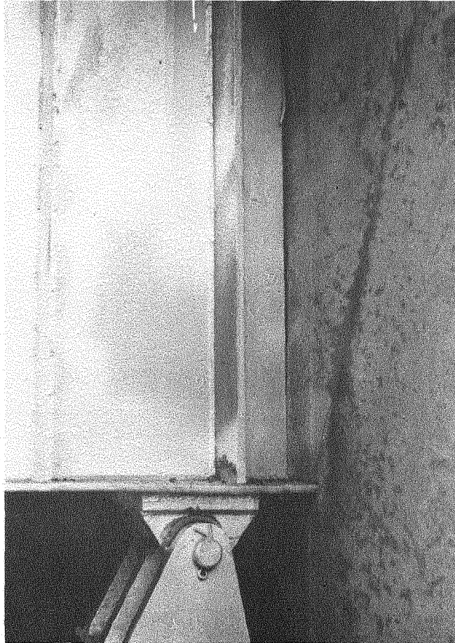
Fig. 2-15. Evidence of extensive movement of abutment headwall
