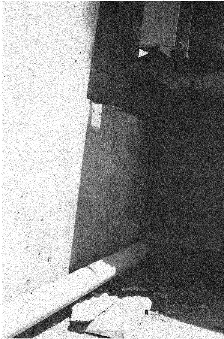
Fig. 2-13. Evidence of a minor movement of the abutment headwall
