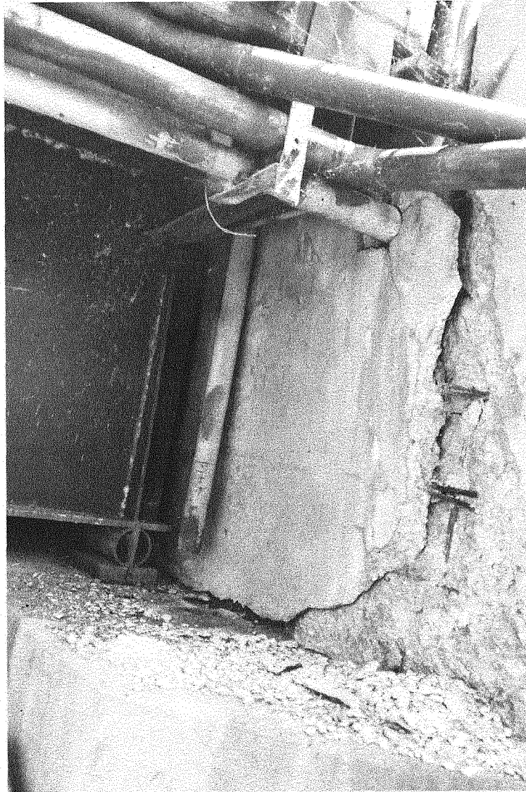
Fig. 2-18. An abutment headwall showing extensive cracking
