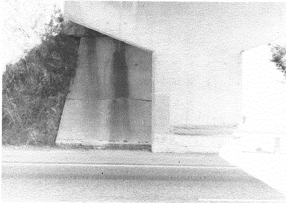
Fig. 2-10a. A slope protection structure showing moderate cracking
