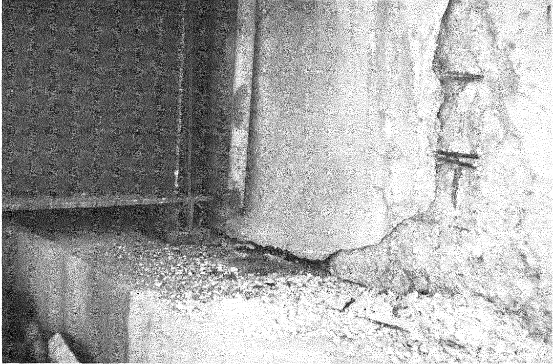
Fig. 2-19. Expansion device showing minor tilting
