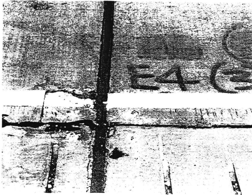
Figure 16. Corner Punchout Above Dowel Bar.
