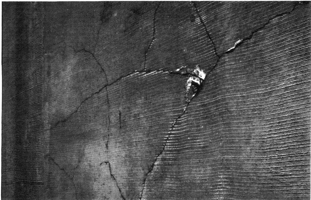
Figure 10. Severely Cracked Section(close-up).
