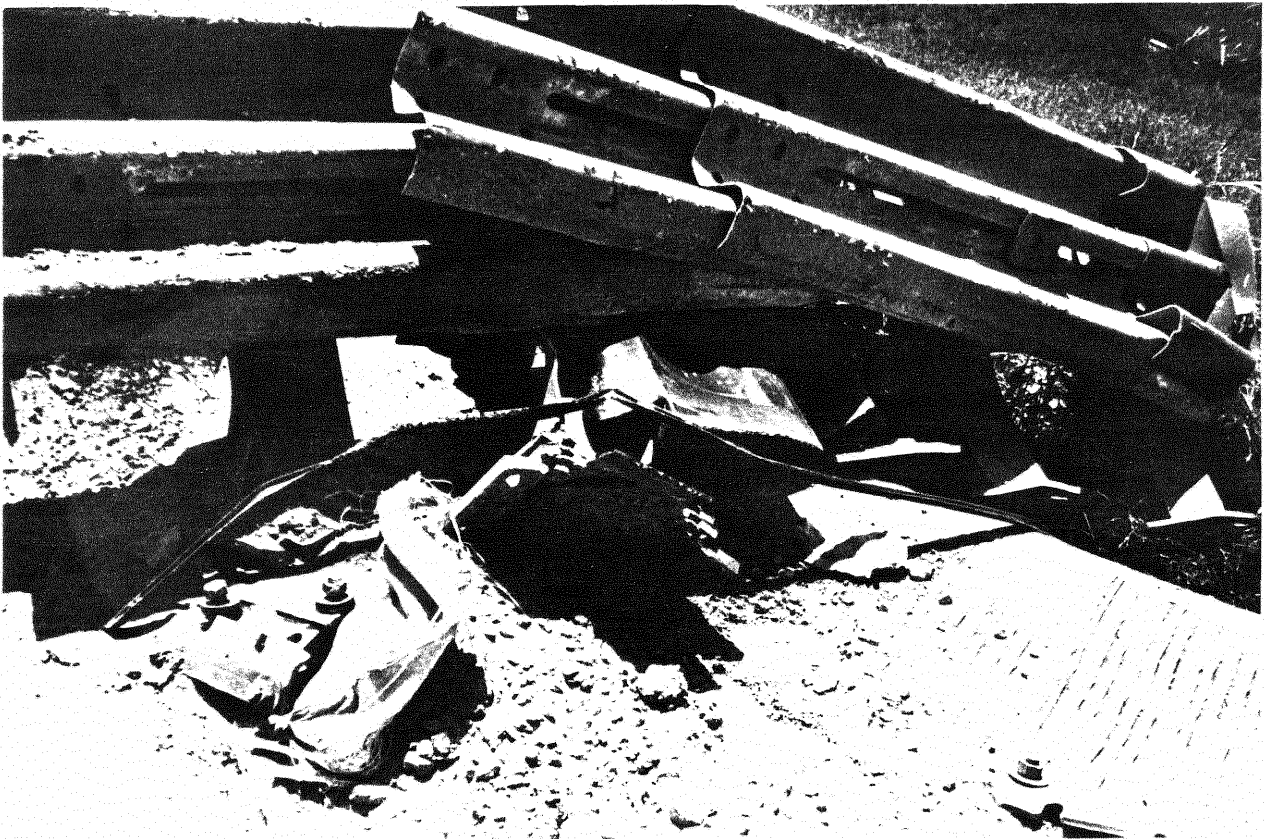
Figure 12. SENTRE unit after impact, unit generally performed as intended, but anchor bolts were pulled out of slab.
