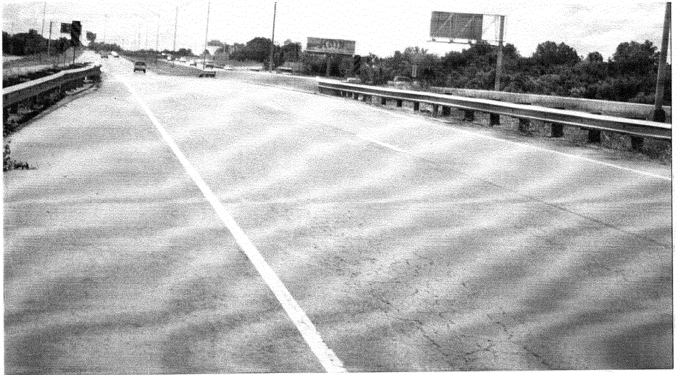
Figure 3. Cracking in outside lane, Novophalt Modified Asphalt Cement Binder section.
