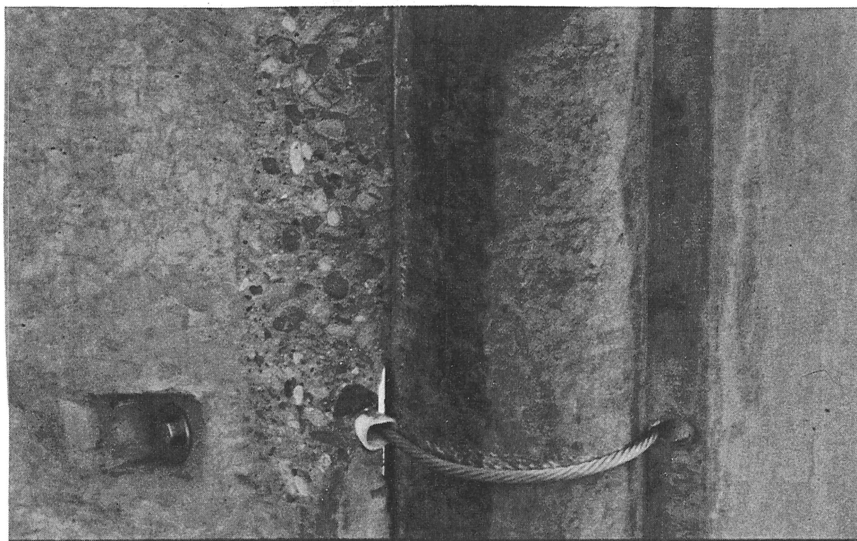
Figure 16. Spall Along Edge of Panel and Break Along Connector Assembly Channel.
