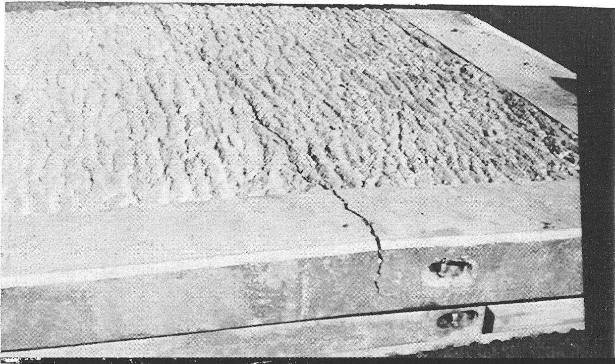
Figure 18. Panel cracked due to misaligned supports during stacking.
