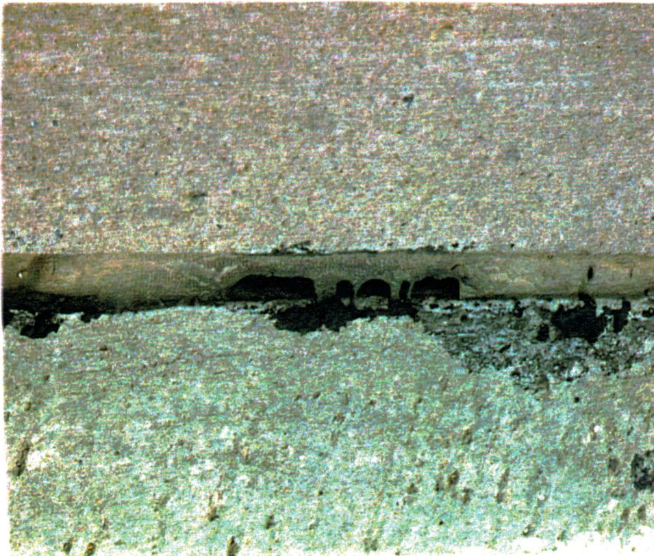
Figure 21. Cohesion Failures in Edge Line Joint.
