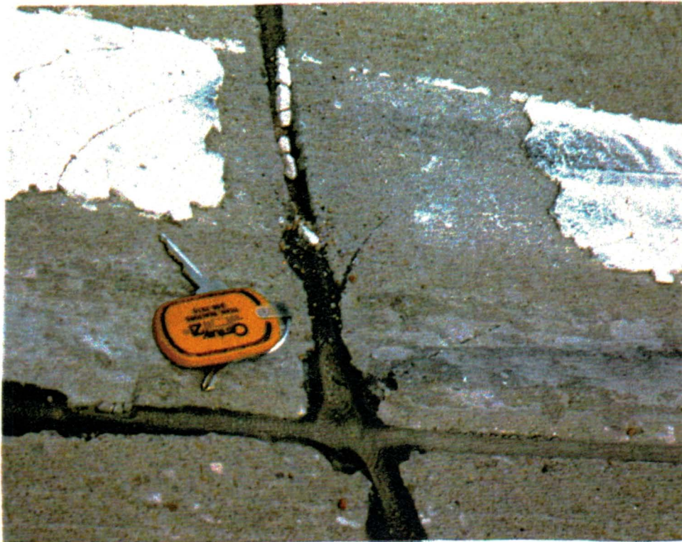
Figure 13. Sealant Dropped into Joint Due to Adhesion Failure on Both Sides.
