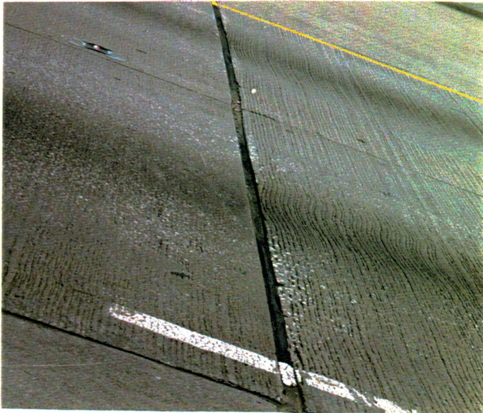
Figure 23. "Polished" Sealant in Wheel Path.
