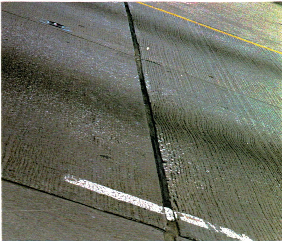
Figure 20. Expansion Joint Sealed with 890-SL with Adhesion Failures in Wheel Paths.
