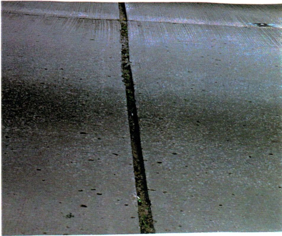
Figure 18. Expansion Joint Formerly Sealed With Hot Pour Sealant.
