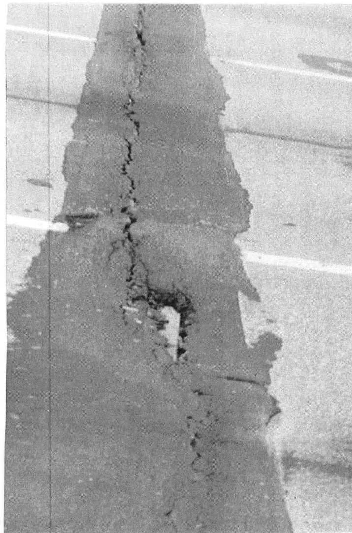
Figure 12. Spalls at Edge of Unit and Along Crack, March 4, 1993
