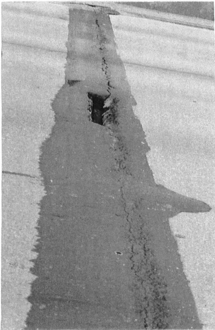
Figure 13. Hole through BJS, Part of Bridge Plate Missing, March 4, 1993.
