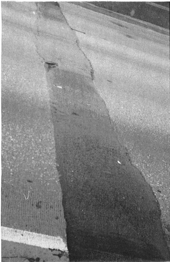
Figure 11. Spalling at edge of BJS Unit, March 4, 1993
