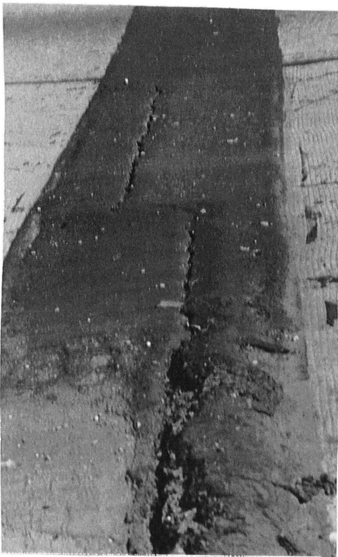
Figure 7. Cracked BJS Unit, 7-10-92.
