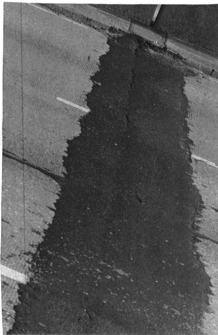
Figure 8. Cracked BJS Unit, 7-10-92.
