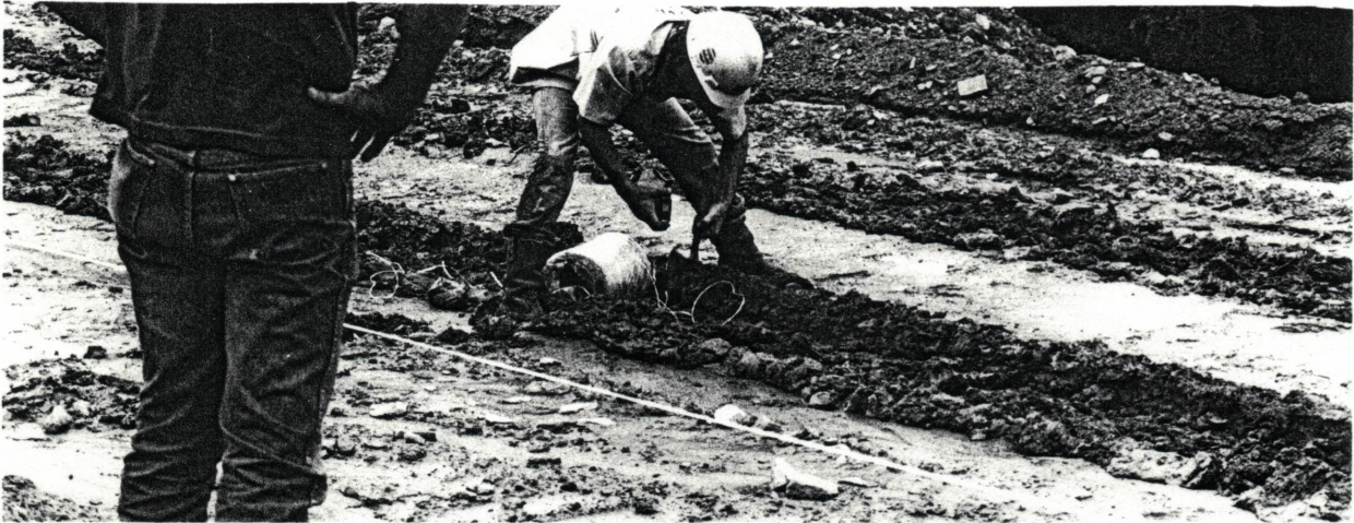
A taught string marks this line of construction on US 69 in Pittsburg County.
