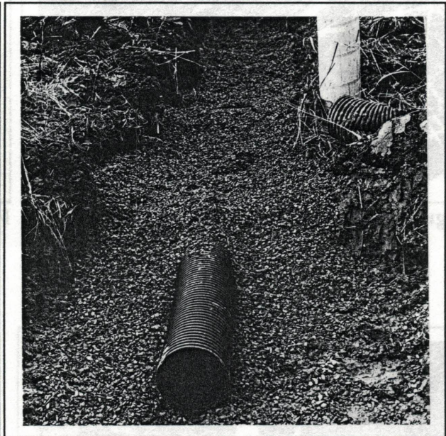
Figure 27 Chips surrounding new outlet.
