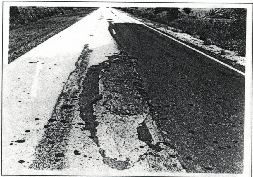
Figure 3 Water related pavement damage.
