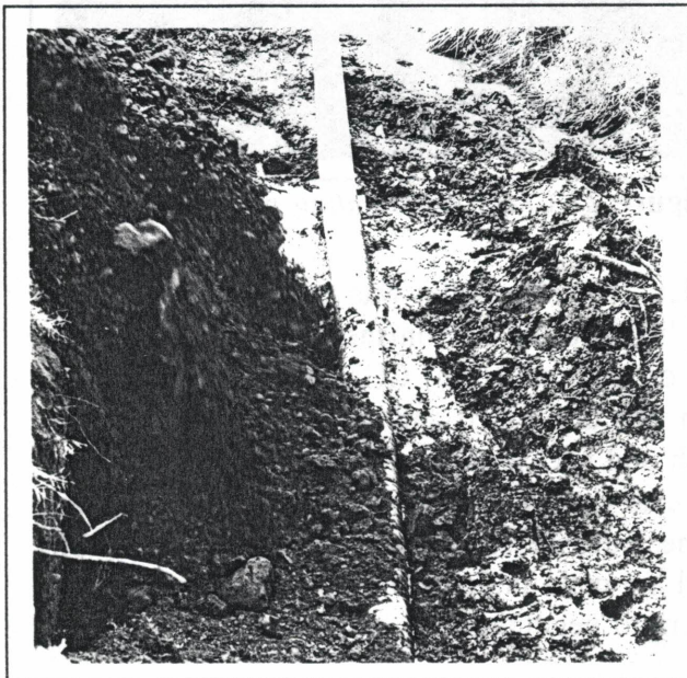
Figure 30 Pipe sliding off center support.
