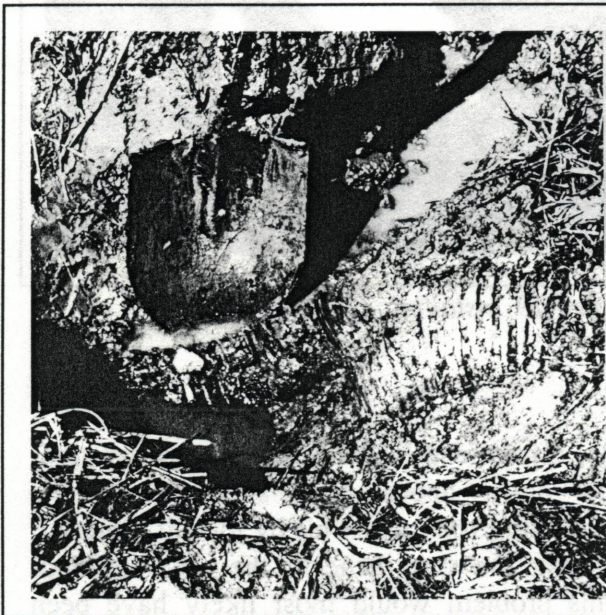
Figure 26 Damaged drain pipe.
