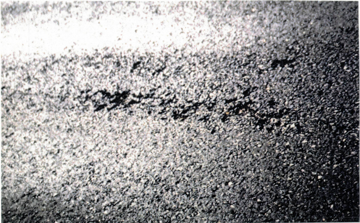
Figure 21. Ravelling of Aggregate From Surface Course.
