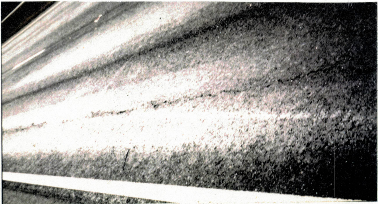
Figure 19. Typical Cracking in AC-30 Section.
