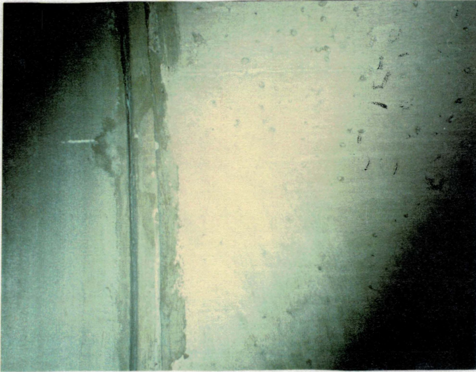
Figure 8. RCP Joint Patched With Mortar.
