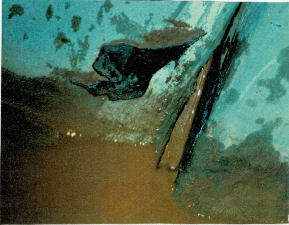
Figure 6. Leaking Joint in 2.4 m (96 in) RCP.
