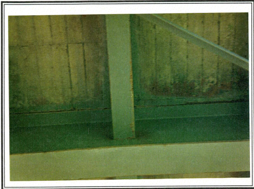
Figure 1: Rust at ends of Beams - McCurtain County .
