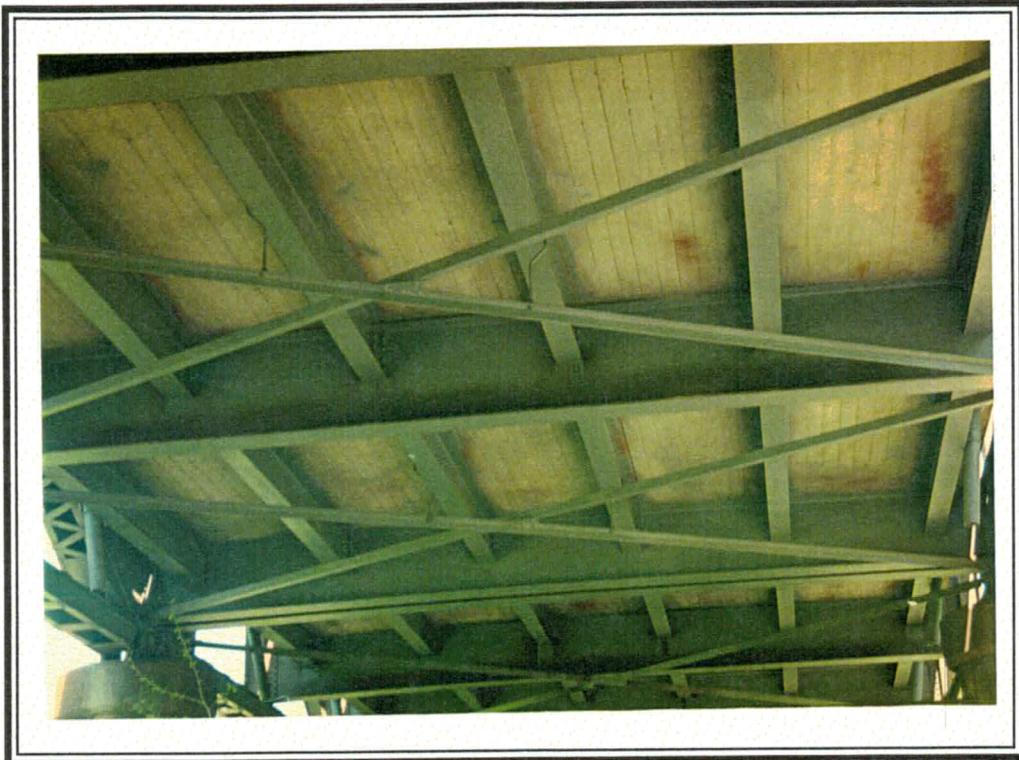
Figure 3: Rust along Bottom of Web - McCurtain County .
