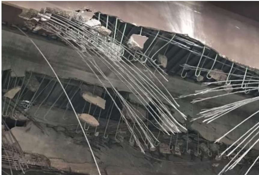
Figure 2.2 Rockville Road Bridge Damage (INDOT, 2017)
