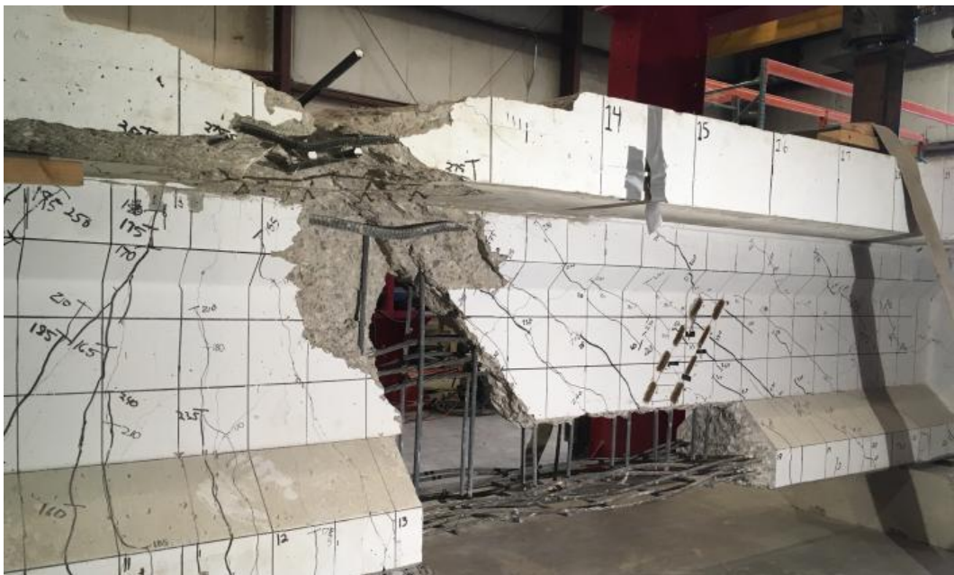
Figure 5.23 Further Damaged Concrete Uncovered During Demolition
