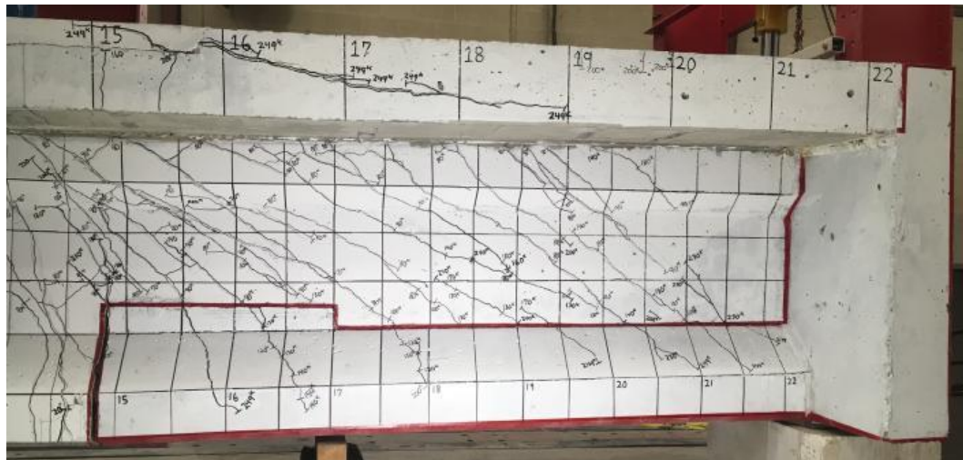
Figure 6.7 Extent of Damage for South End Repair
