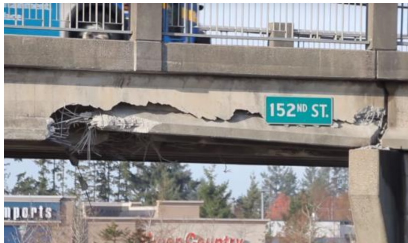
Figure 1.1 Impact Damaged, Prestressed Concrete Bridge (Greenizan, 2017)
