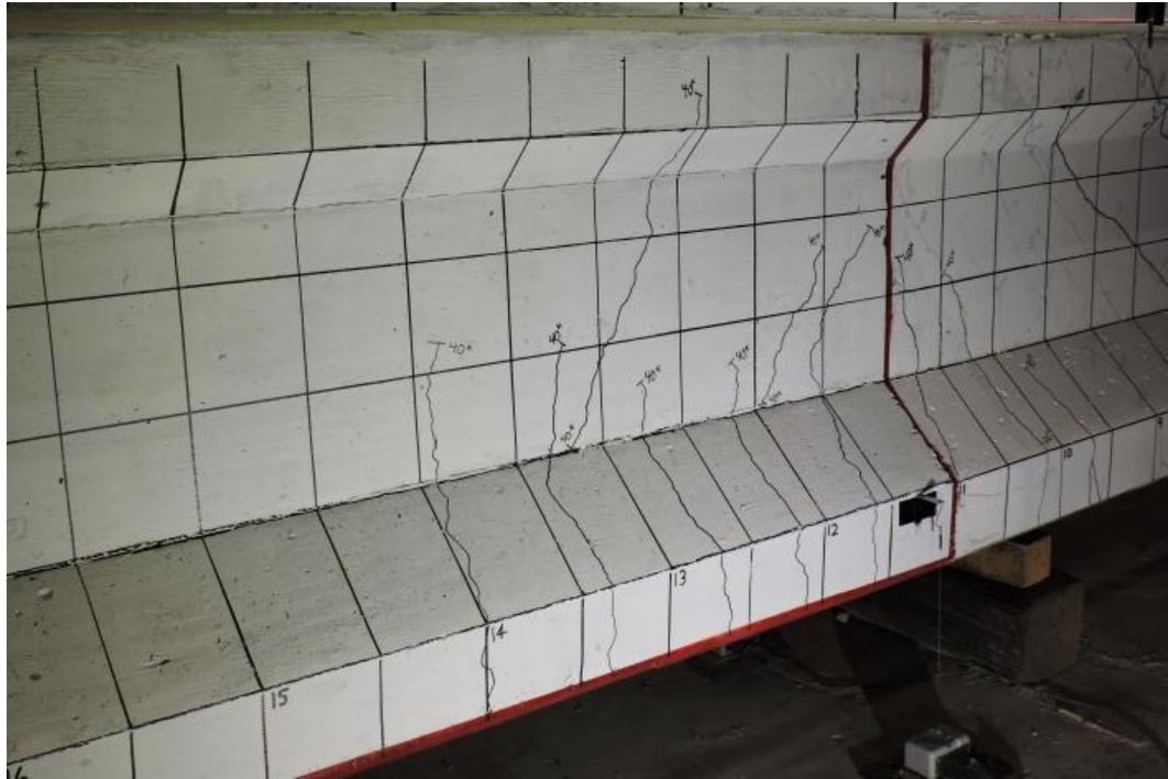
Figure 6.11 First Cracks in the Repair Zone
