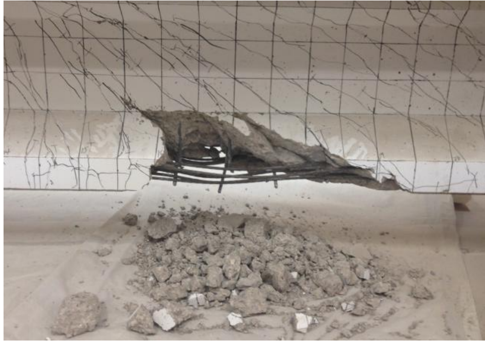
Figure B.1 Loose Concrete Removed From South End With Hammer
