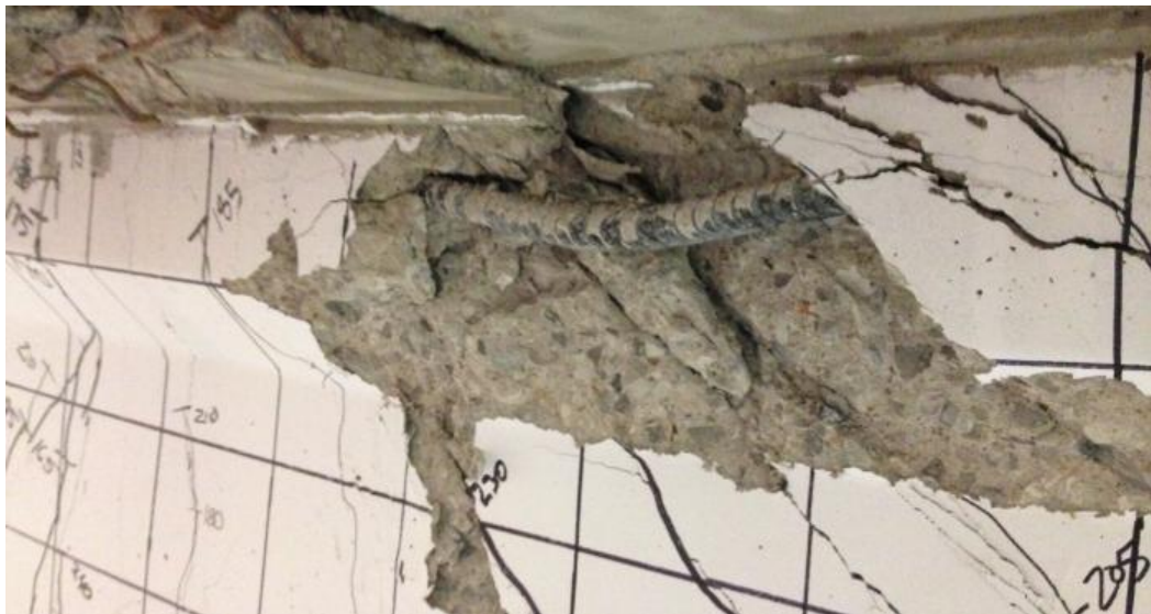
Figure 4.9 Buckled, Longitudinal No. 8 Reinforcing Bar in the Top Bell of the Girder
