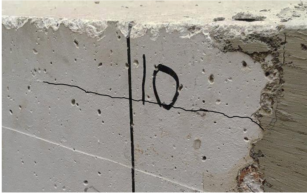
Figure 6.13 Delamination of Wearing Layer During Repair Testing
