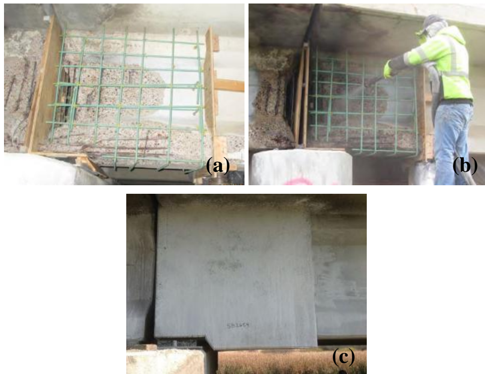
Figure 2.1 University of Minnesota Shotcrete Repair Project; (a) Added Repair Reinforcing; (b) Shotcrete Application; (c) Completed In Situ Repair (Shield, 2018)
