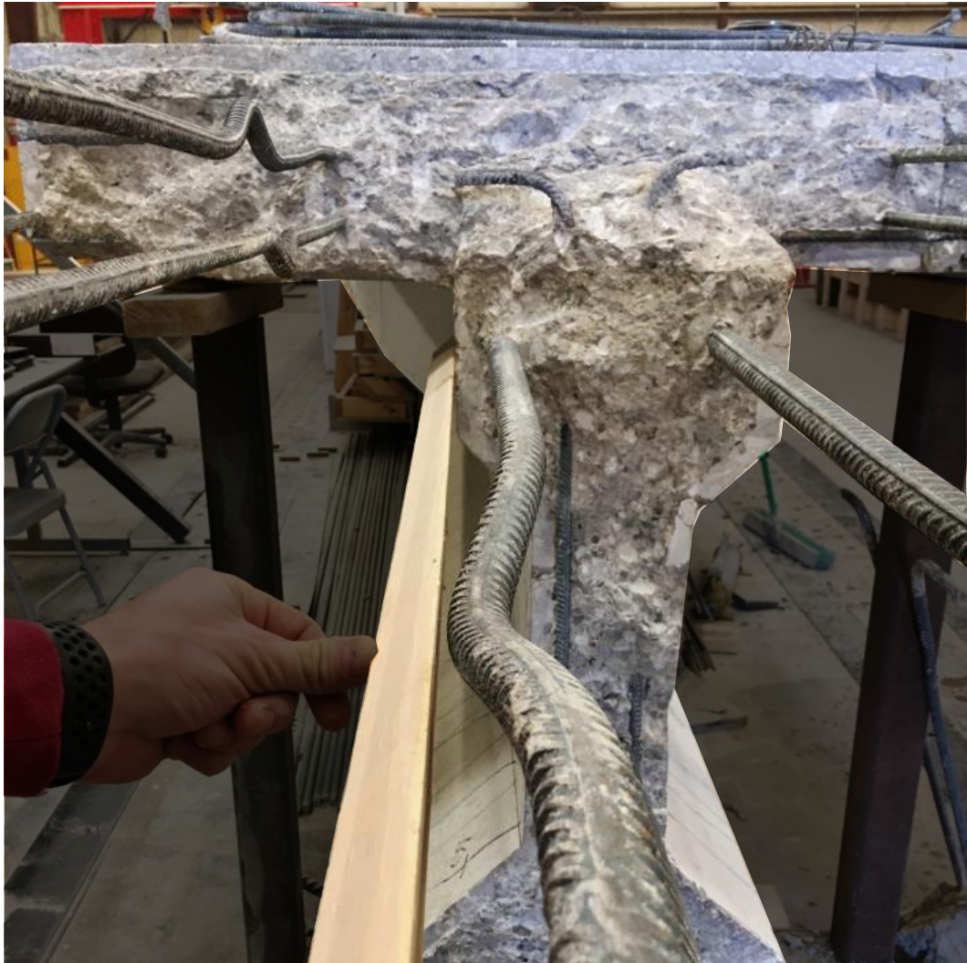
Figure C.3 Bent Longitudinal Reinforcing of North End Repair
