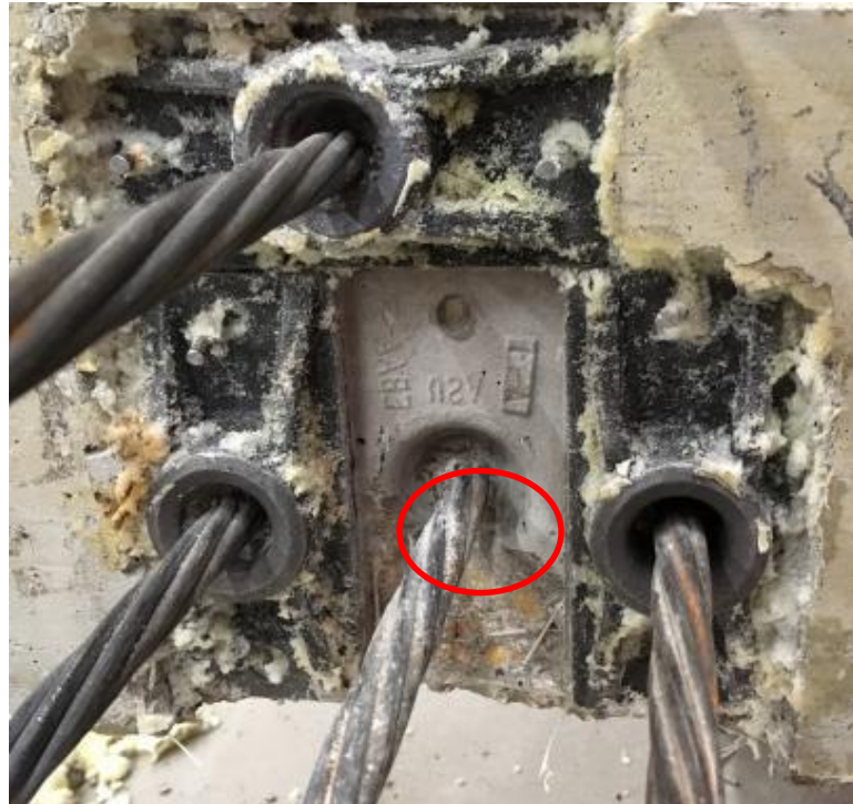
Figure 5.19 Damaged Area After Removal of Anchor Plate
