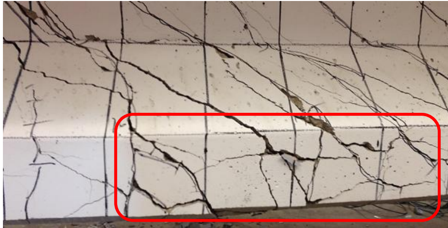
Figure 4.5 Shear & Horizontal Cracking in the Bottom Bell
