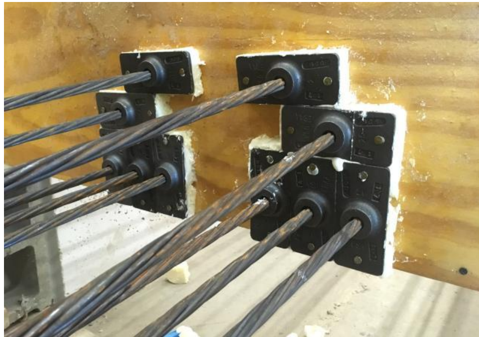
Figure C.2 Post-Tensioning Anchorage Installed to Formwork With Insulating Foam to Seal the Backside
