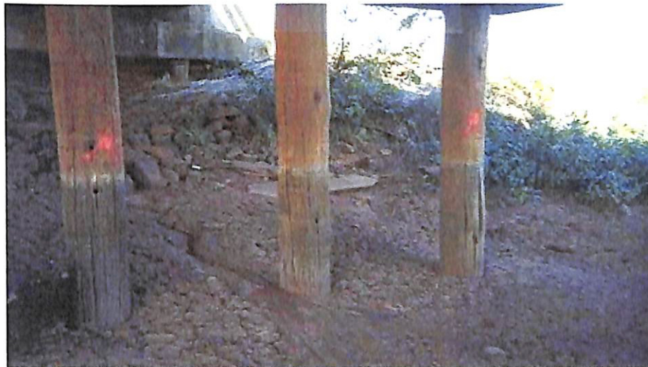
FIG. 1.1. Decayed Timber Piles in Service
