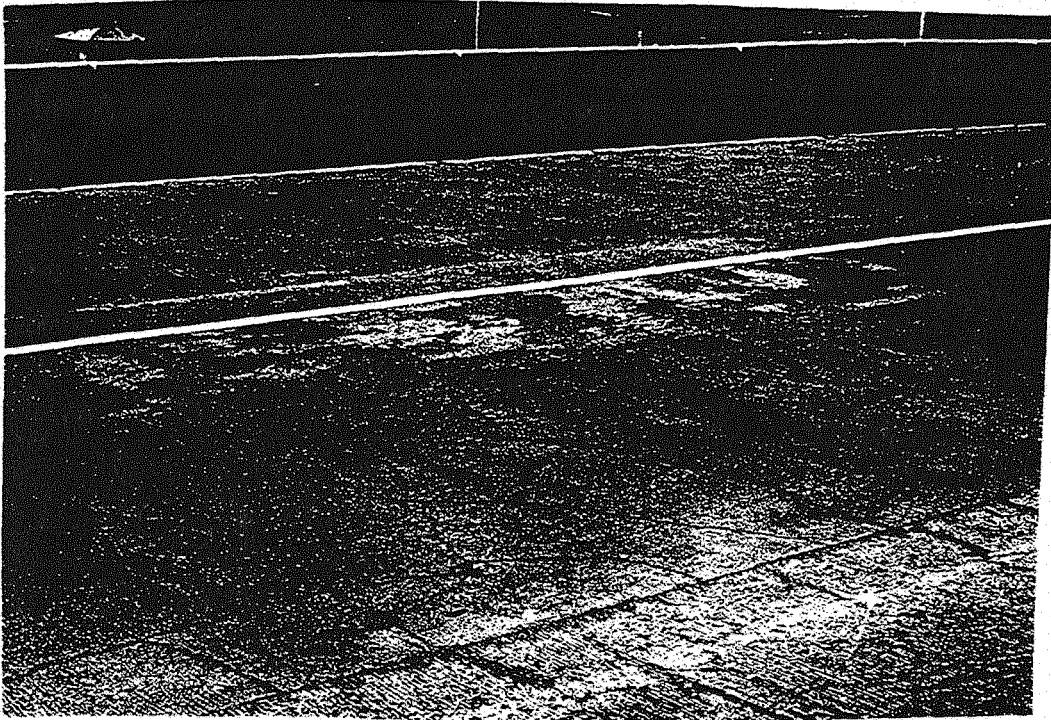
Figure 4. Cracks in Pavement.
