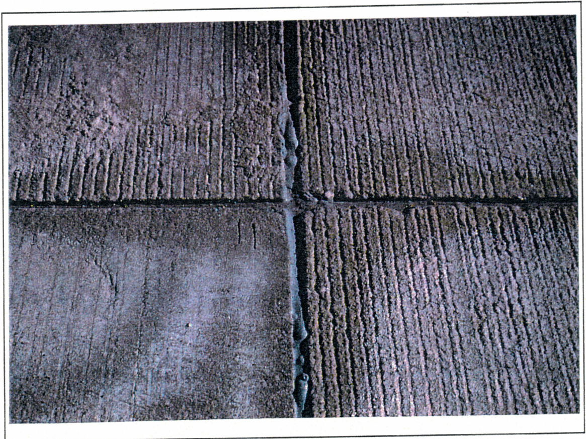
Figure 7. Bubbles in sealant
