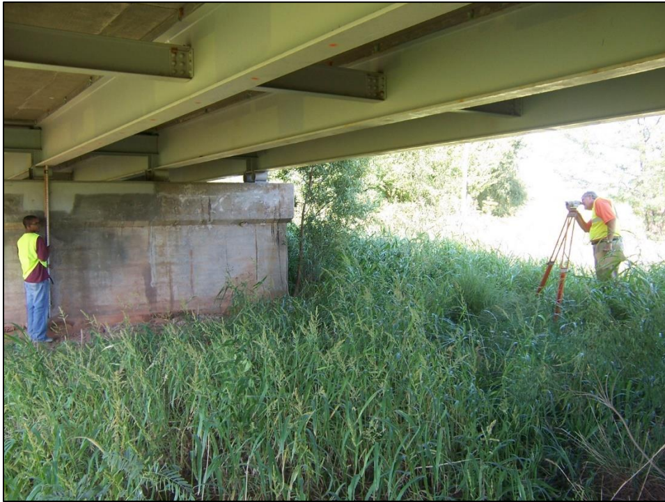
Figure 31: Elevation readings on the bottom of the steel girder at a pier for SH 14
