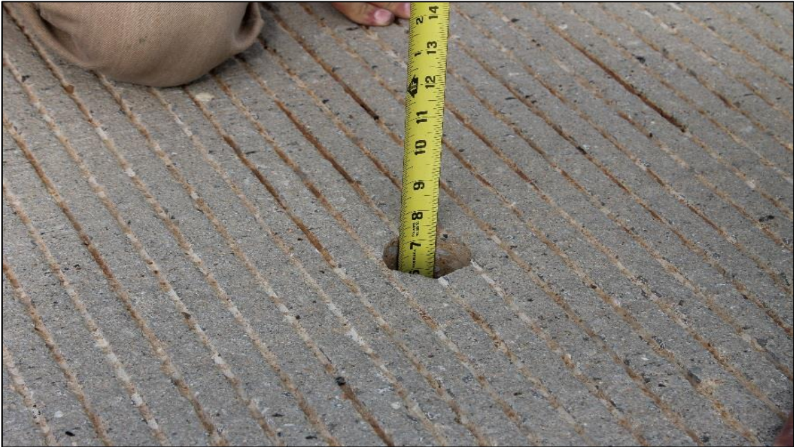
Figure 63: A pre-existing core hole discovered in span 2 of SH 14
