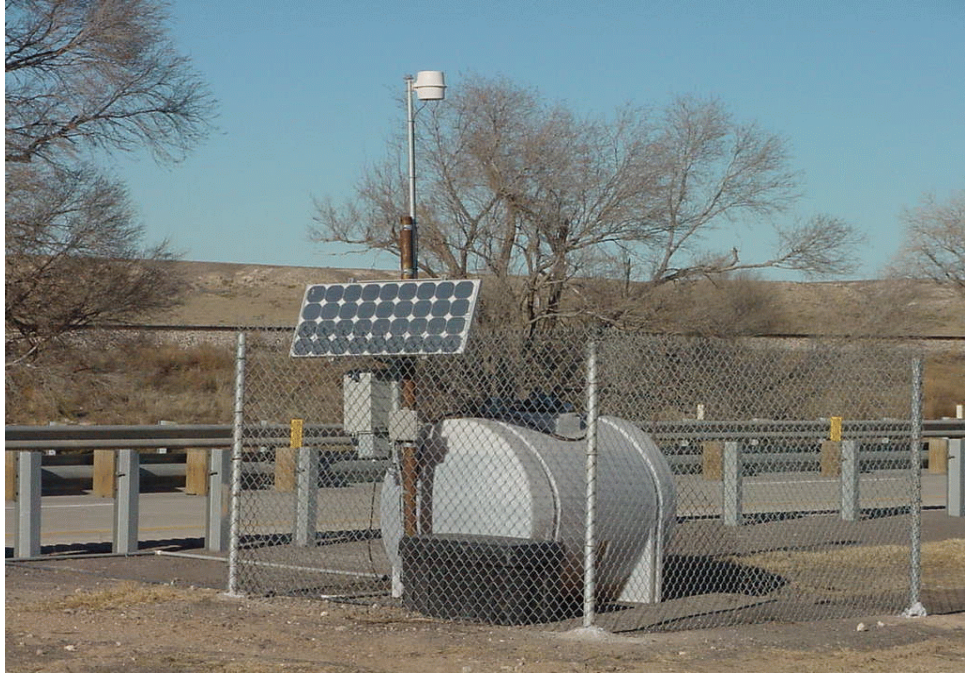
Figure 8. Solar Powered Fixed Anti-icing Tracking System Master Station
