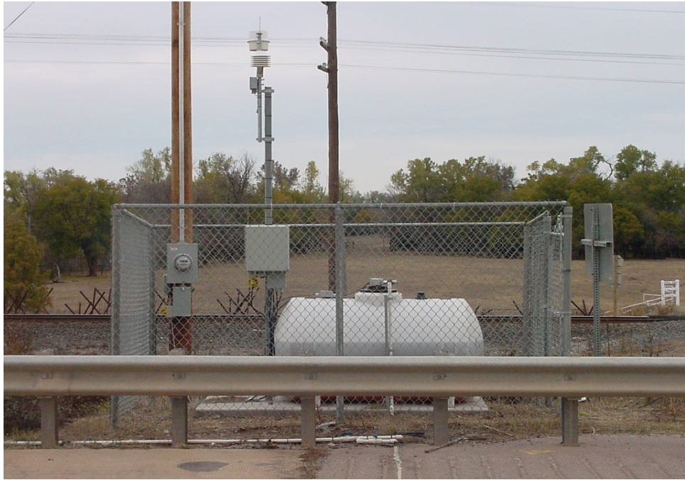
Figure 7. Electrical Powered Fixed Anti-icing Tracking System Master Station
