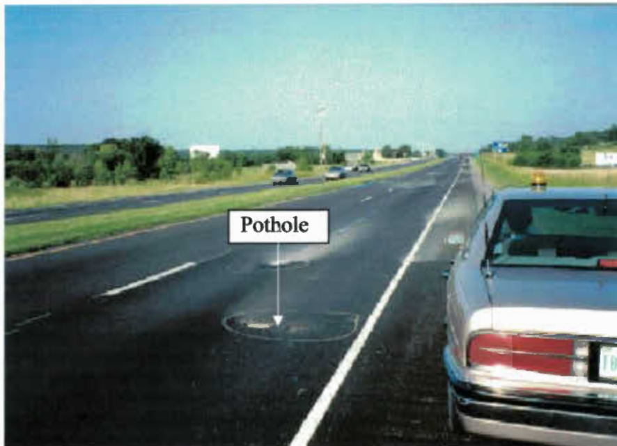
Figure 1.2 Potholing in the Inside Wheel Track of Slow Lane (Will Rogers Parkway, Oklahoma)
