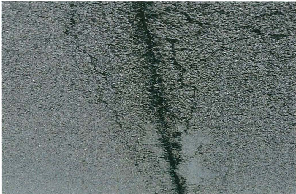
Figure 2. Centerline raveling and cracking.
