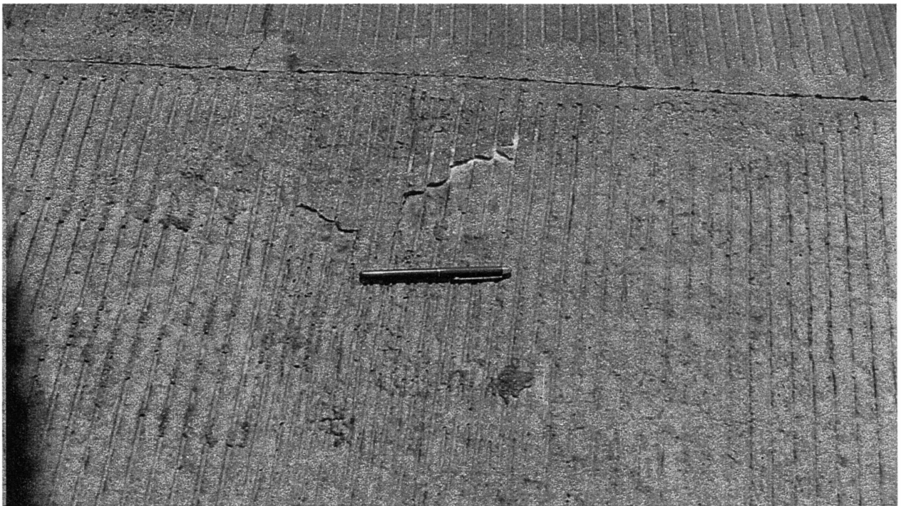
Figure 6. Longitudinal Construction Joint Crack.
