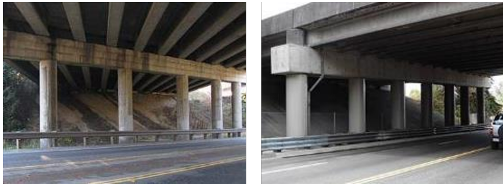
Figure 2.2: Seismic retrofit for bridge using steel jackets in columns. Left: before retrofit; right: after retrofit.
