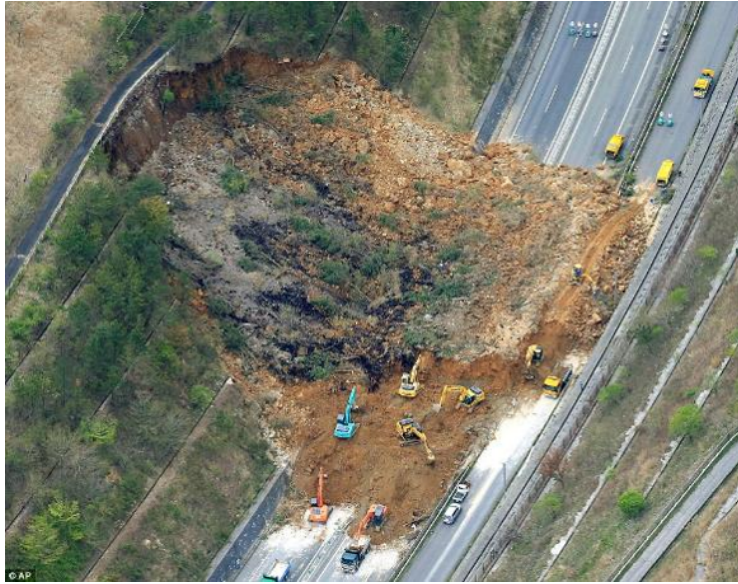
Figure 2.1: Obstruction in highway.
